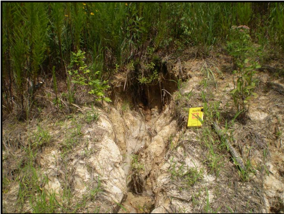
SPA8 – Erosion on left bank @ station 334+00 (UT3)
