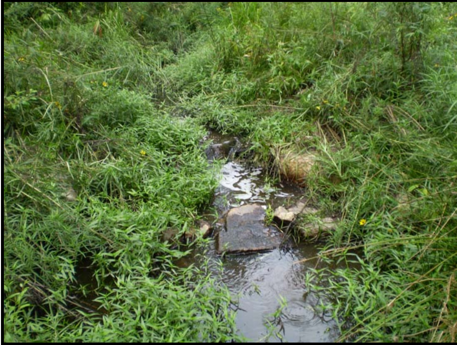
SPA3 – Piping around header rock on rock A-vane @ station 134+40 (UT1-A)
