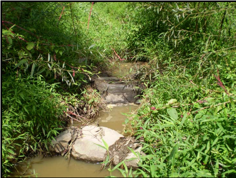
SPA4 – Piping around header rock on rock A-vane @ station 211+00 (UT2)
