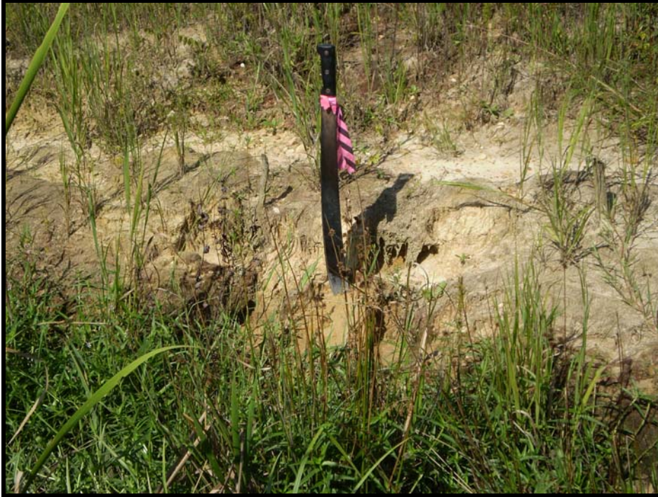
SPA1 – Erosion on right bank @ station 107+15 (UT1-C)
