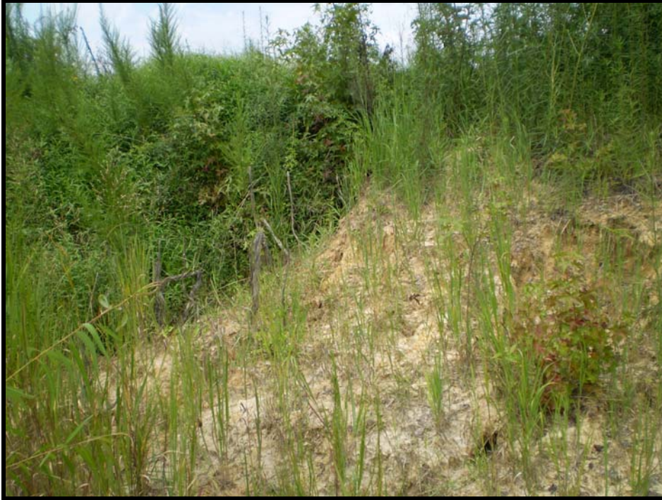
SPA7 – Erosion on left bank @ station 330+50 (UT3)
