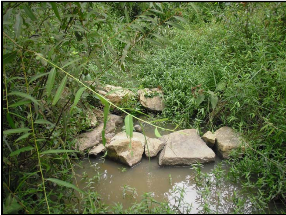
SOA2 – Piping around header rock on Rock A-vane at Sta. 134+50 (UT1-A)
