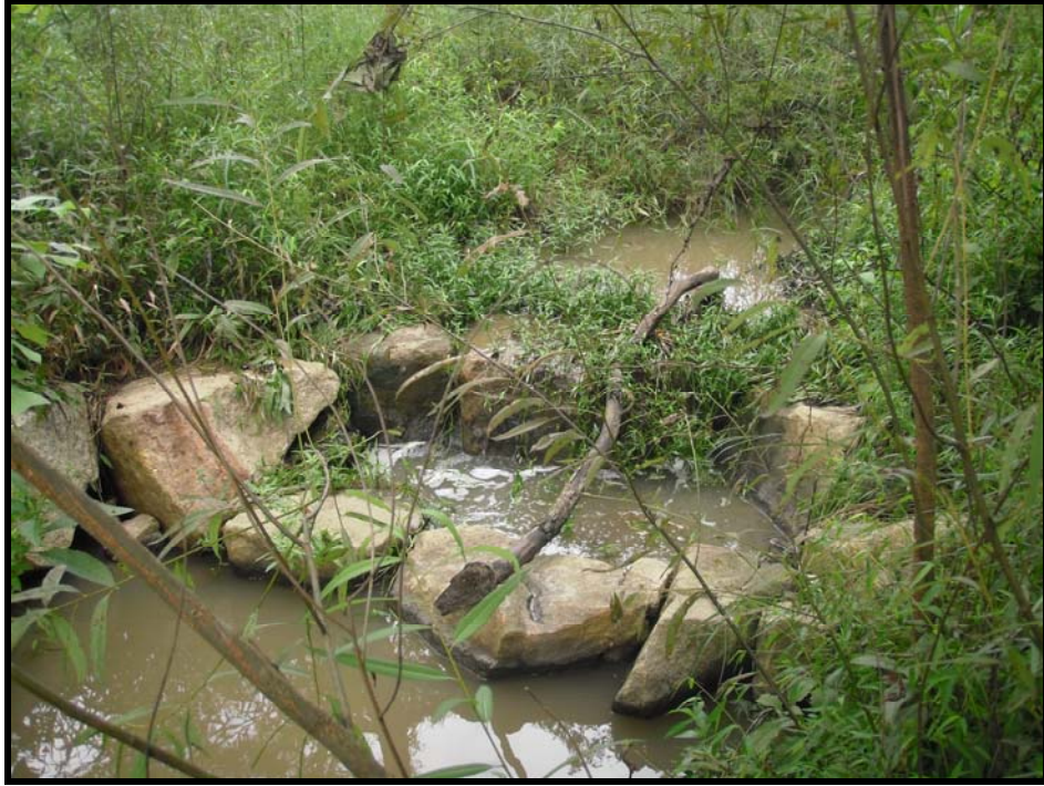
SOA1 – Piping around header rock on Rock A-vane at Sta. 133+30 (UT1-A)
