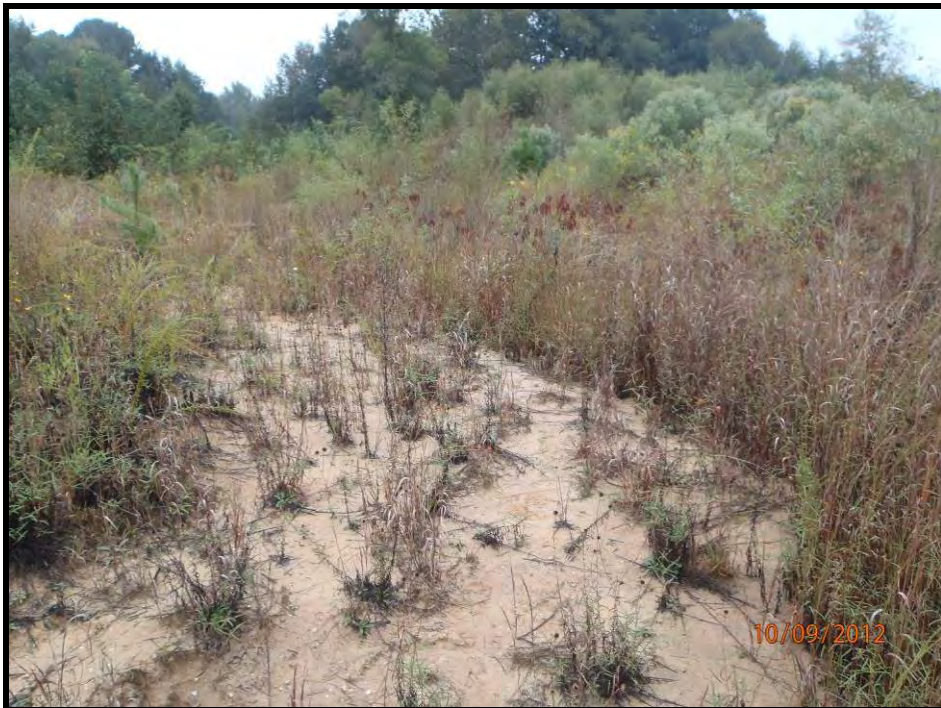
SOA3 – Sparse vegetation on left and right banks at Sta. 304+30 – 304+50 (UT3)
