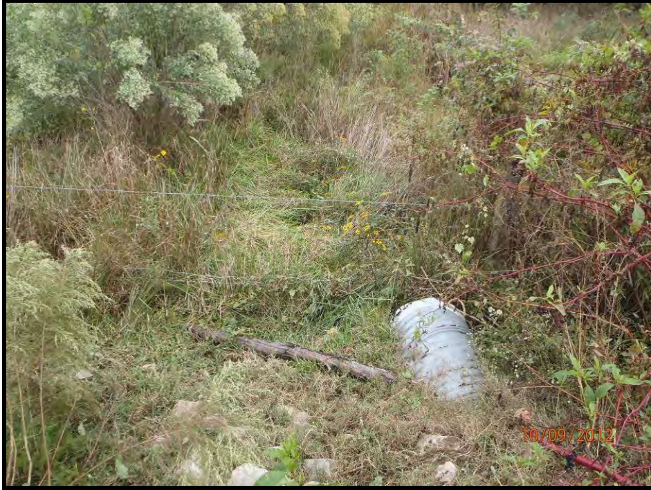
SOA2 – Easement fencing is loose at Sta. 119+50 (UT1-B)
