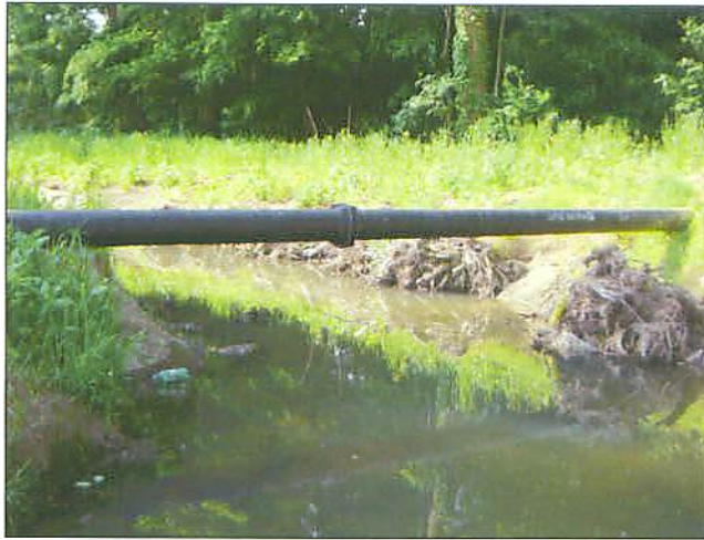
PP#36B R2 Rock Vane #5, newly installed aerial sewer and Root Wad Cluster #6
