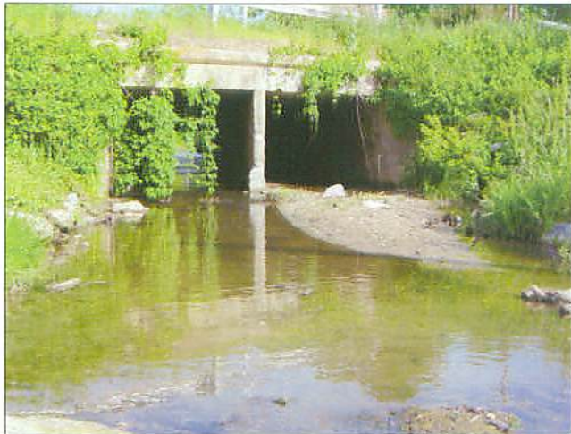
PP#18A R2 upstream view of stabilized culvert from invert of Double Drop Cross Vane #1
