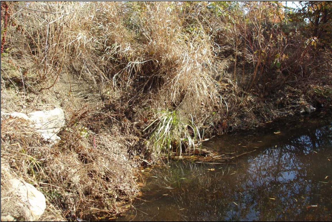
SP3 - Bank erosion has occurred behind coir matting. Photo taken near Station 19+50. 11/16/07 - MY 03
