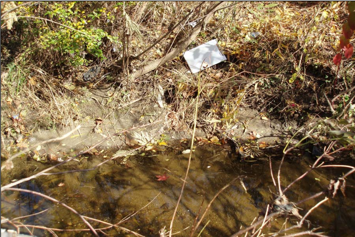
SP1 - Bank erosion. Photo taken near Station 11+15. 11/16/07 - MY 03
