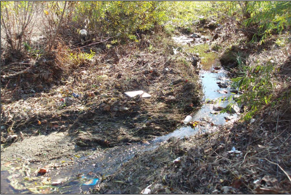
SP5 - Stream aggradation over constructed riffle causing narrowing of the channel. Photo taken near Station 21+60. 11/16/07 - MY 03
