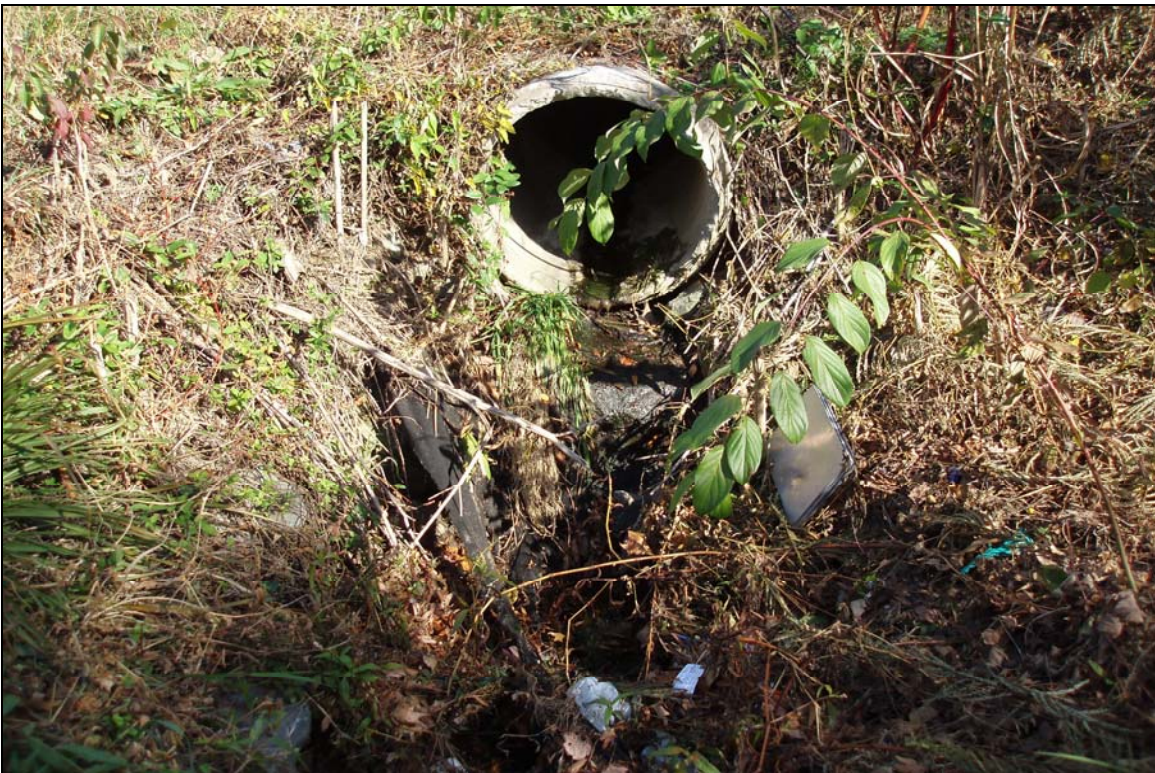
SP2 - Step pool structure failed, de-stabilizing stormwater drain outlet. Photo taken near Station 19+00. 11/16/07 - MY 03
