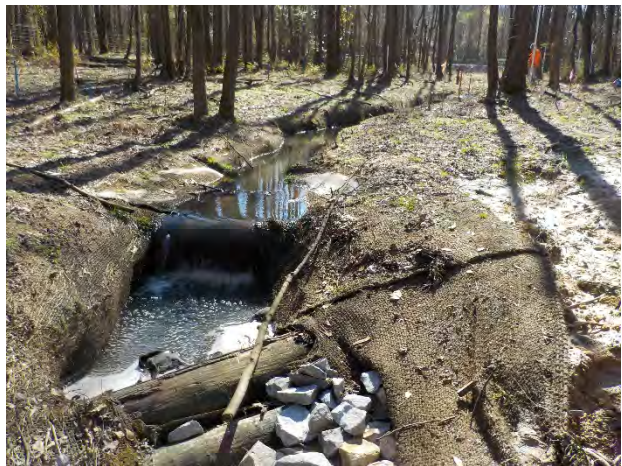
SPA6- Loose structure and bank erosion- UT4 @ Sta 10+25 to 11+00
