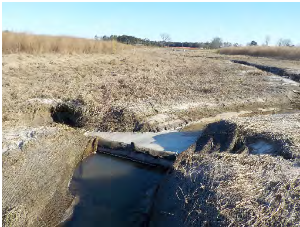
SPA5- Loose grade control structure- UT2 @ Sta. 26+25
