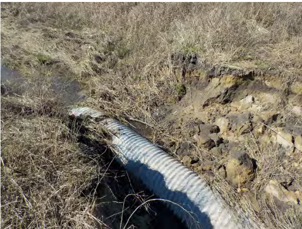
SPA7- Failing Crossing- UT8 @ Sta 4+07 to 4+67
