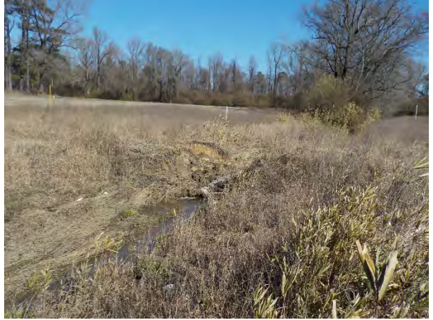
SPA7- Failing Crossing- UT8 @ Sta 4+07 to 4+67
