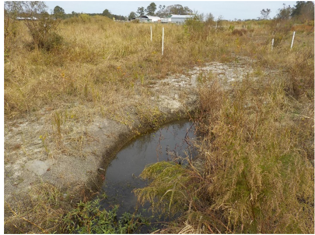
MY1 - SPA2- Bank Erosion and Loose log structures- UT1
