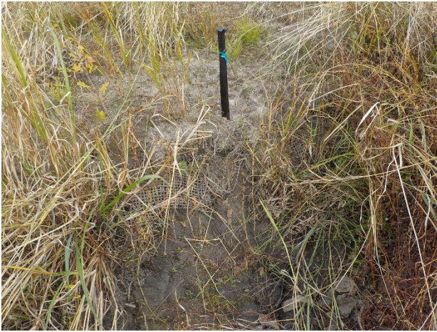
SPA1- Minor Bank Erosion- UT1 @ Sta. 12+60
