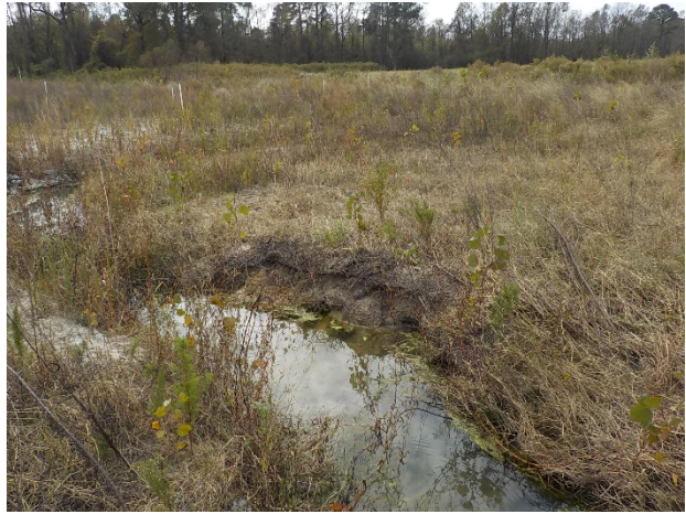
SPA2- Bank Erosion and Loose matting- UT2 @ Sta. 27+00
