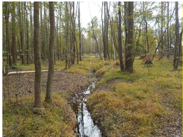
MY1 - SPA6- Loose structure and bank erosion- UT4
