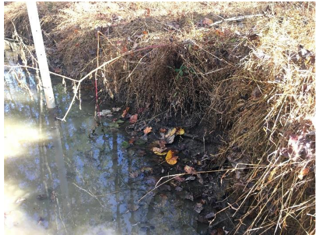
SPA2 – Minor Bank Erosion UT 4 @ Sta. 5+60 to 7+00
