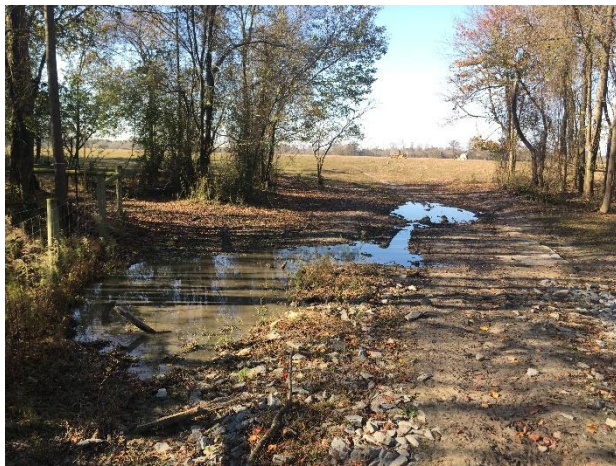
SPA3 – Ponding on Road UT 4 @ Sta. 8+47 to 8+67
