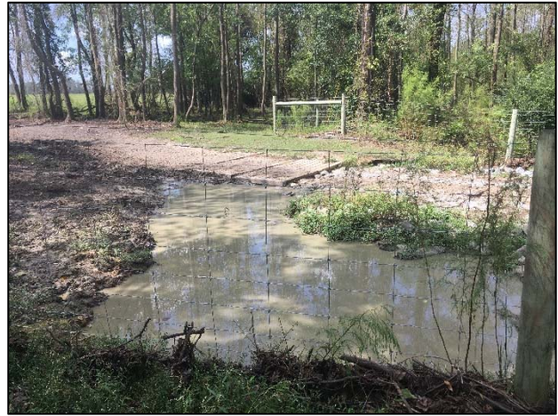
SPA2 – Ponding on Road UT 4 @ Sta. 8+47 to 8+67*
