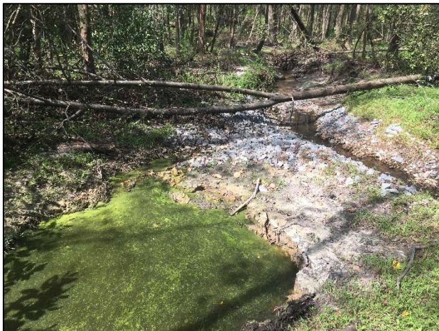
SPA3 – Relic Channel Floodplain Plug Subsidence UT4 @ Sta. 8+75 to 11+03*
