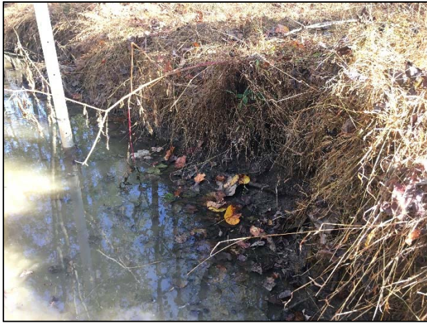
SPA1 – Minor Bank Erosion UT 4 @ Sta. 10+10 to 10+30
