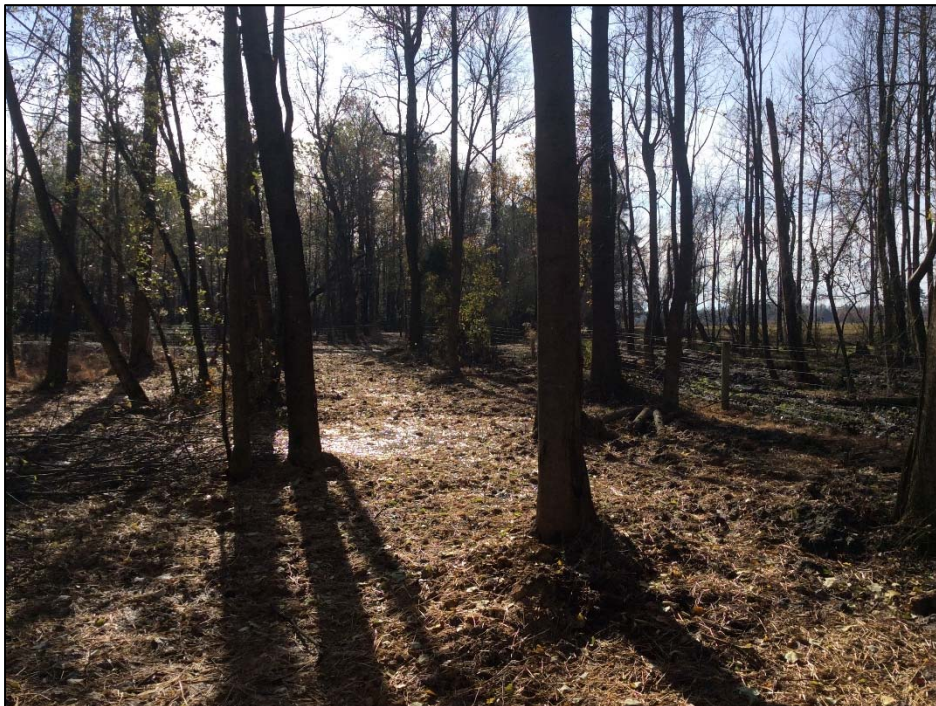
SPA3 – Relic Channel Floodplain Plug Subsidence UT4 @ Sta. 8+75 to 11+03 (Photo of repair - December 2018)
