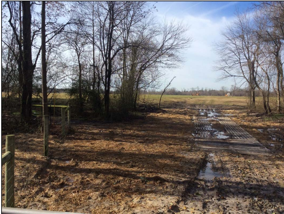
SPA2 – Ponding on Road UT 4 @ Sta. 8+47 to 8+67 (Photo of repair - December 2018)
