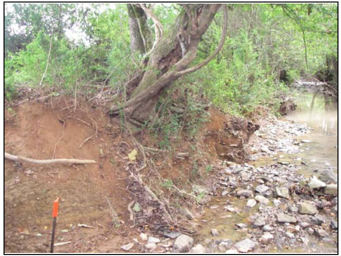
Big Cedar Creek – near center of project. High erodibility and lack of surface protection results in shear, unstable banks.
