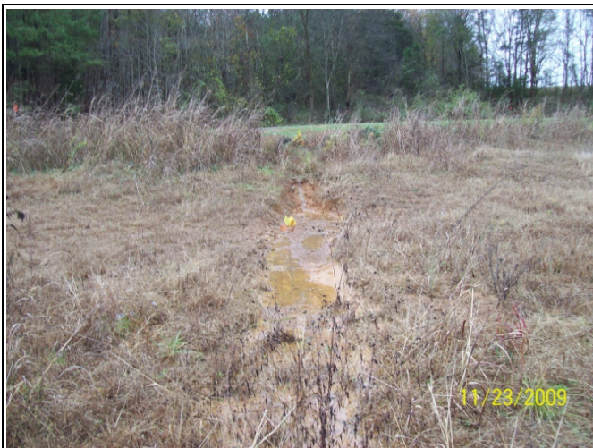
VPA 5 – Bare spot from offsite storm pipe.
