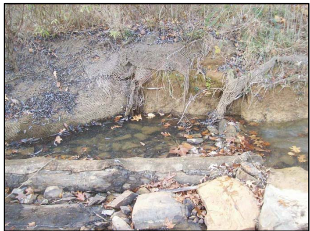
SPA 4 – Erosion/Scour behind log sill
