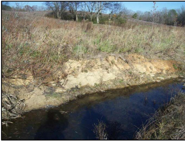
VPA 7 – UT1 Bare Bank loss of matting
