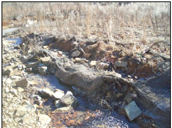
SPA 18 – UT2 Bank Slump
