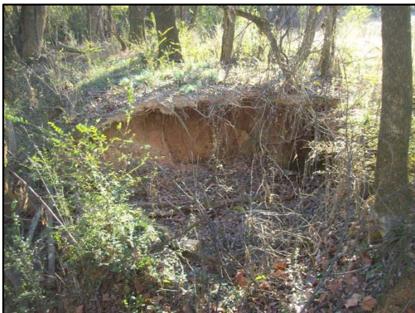
SPA 11 – Bank Sinkhole from up-rooted tree
