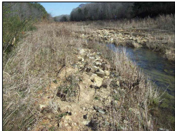
SPA 12 – UT1 Bank scour
