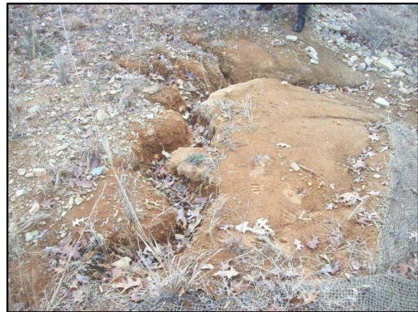
SPA 10 – Bank scour from overland stormwater flow
