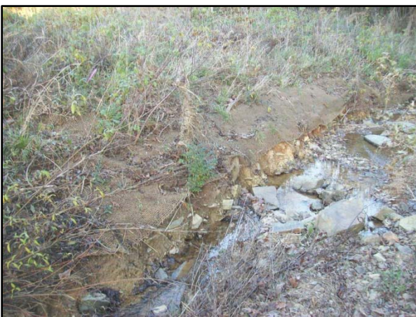
SPA 5 – BCC Toe Erosion from thalweg shift
