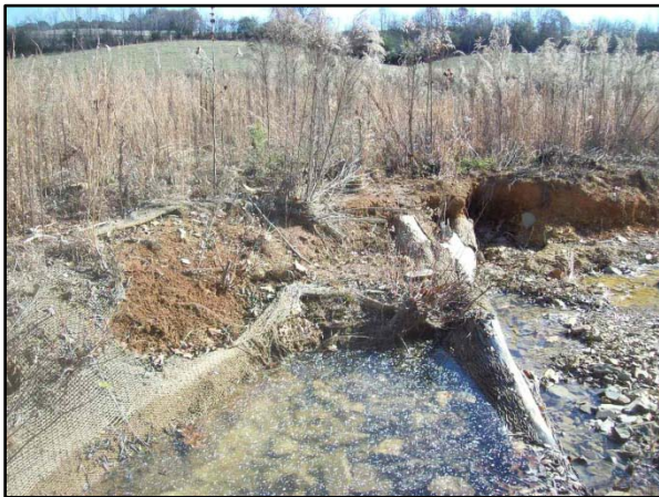
SPA 9 – Log sill set too low
