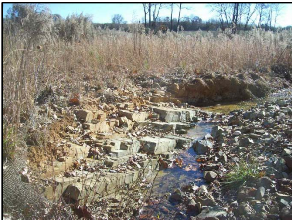
SPA 17 – UT2 Bank scour from lack of vegetation due to poor soils
