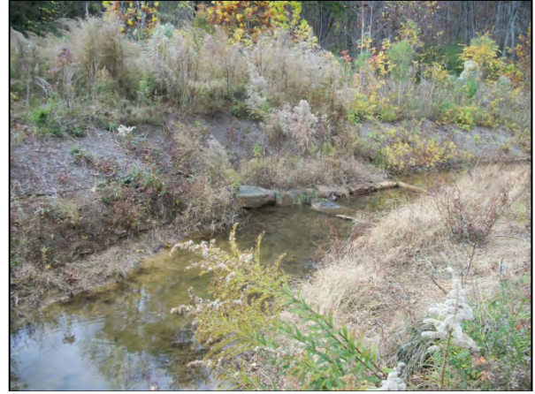
VPA 4 – Bare bank along BCC at Station 29+00 to 29+75, right bank
