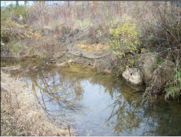
SPA 1 – Minor bank erosion along BCC at Station 24+00, left bank
