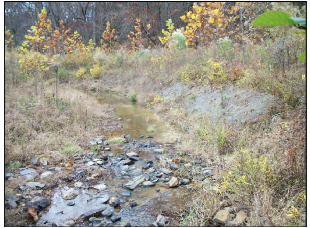
VPA 2 – Bare bank along BCC at Station 26+00 to 26+60, right bank
