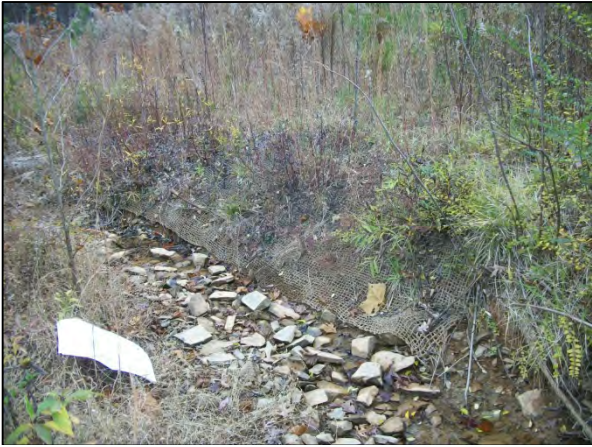
SPA 8 – Minor bank erosion along UT2 at Station 12+30, left bank
