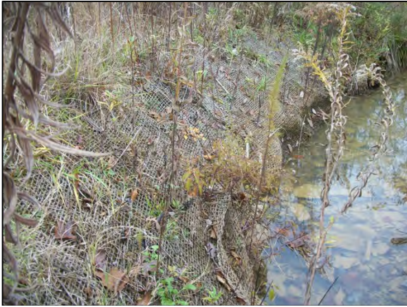
SPA 7 – Minor bank erosion along UT2 at Station 11+30, right bank
