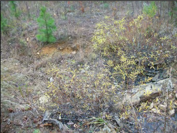
SPA 10 – Bank scour at Station 14+00 on right bank, UT2
