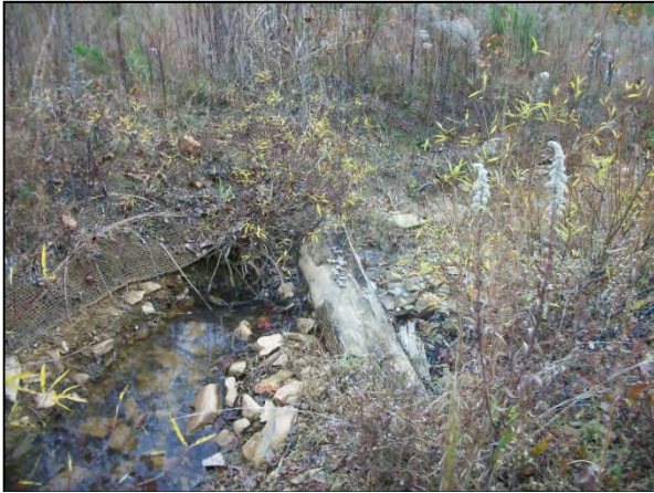
SPA 9 – Minor bank erosion along UT2 at Station 13+75 to 14+30, left bank
