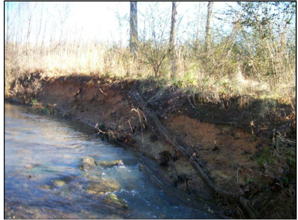
SPA 4 – Bank erosion on left of BCC from Station 46+90 to 47+30
