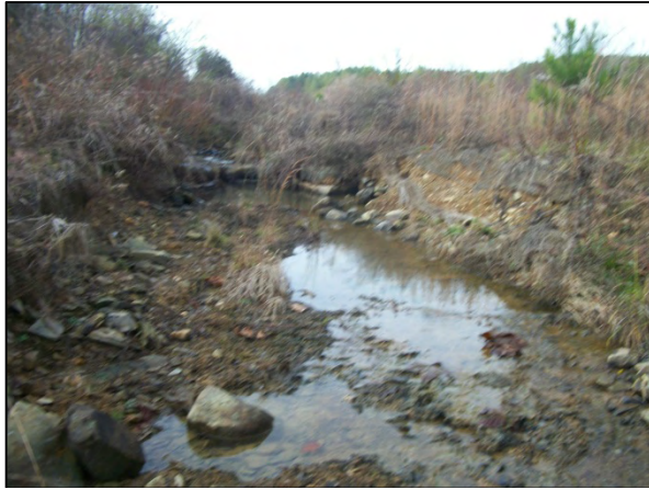
SPA 1 – Minor bank erosion on UT1 at Station 56+60, left bank
