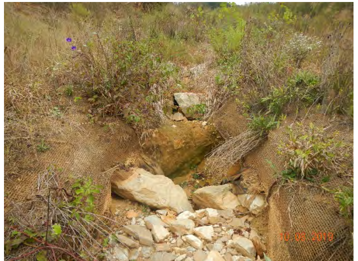
Royster Creek R1 Boulder Sill Failure (Station 806+75) – view upstream (10/8/2019)
