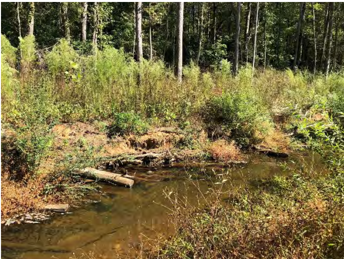
LBHC R2 Bank Scour (Station 316+00) – view downstream (10/8/2019)
