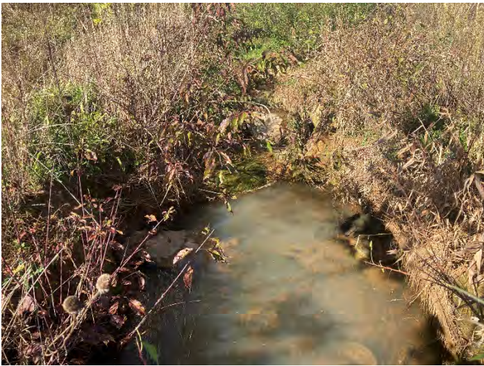
Royster Creek R1 Rock Sill Failed (STA 806+74) – view upstream (10/27/2020)
