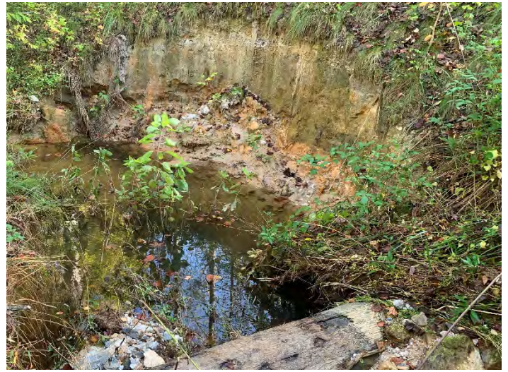
USEC R1 Bank Scour (STA 1005+57 – 1005+75) – view downstream (10/20/2020)
