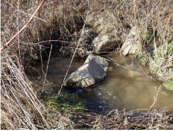
Area in the vicinity of cross-section 2. Water is piping through the boulders.
