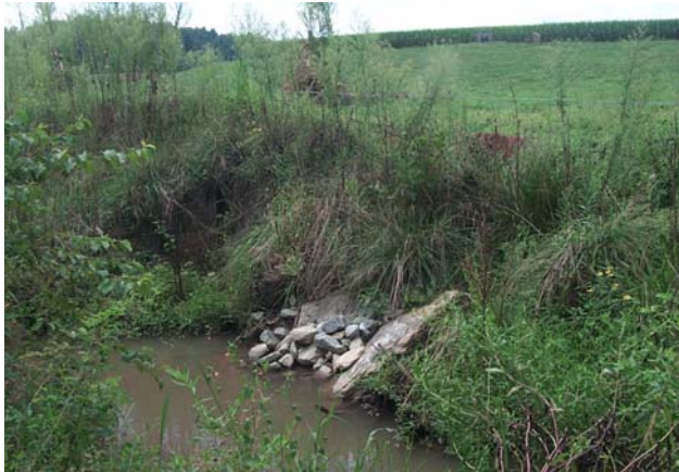
Before stream bank repairs to the left bank above cross-section 3, September 2005.
