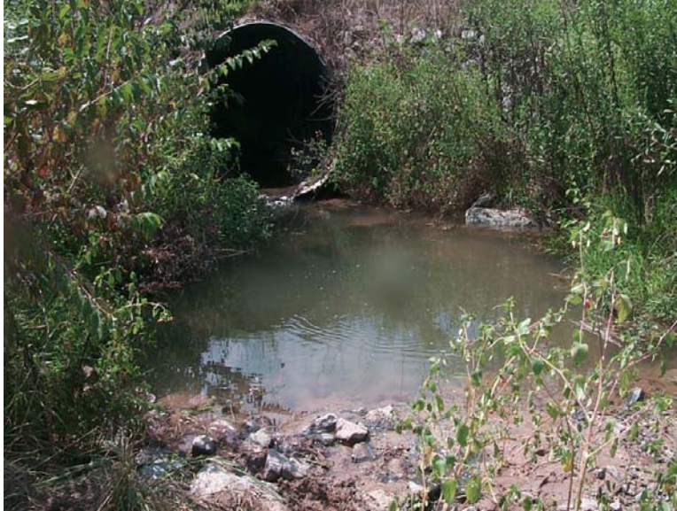
Repositioned boulders and added geotextile fabric to the rock sill in front of the culvert, September 2005.
