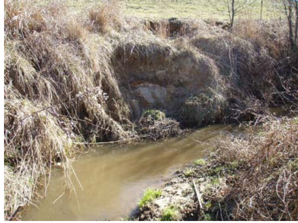
Area between cross-sections 1 and 2, LUS. Banks are sloughing due to overland flow.
