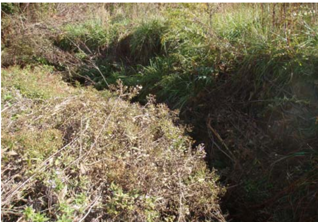
Eroding right bank below cross-section 6, LDS, November 2008.
