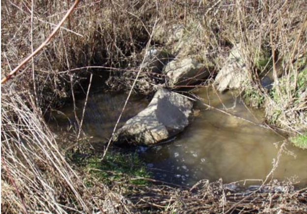
Area in the vicinity of cross-section 2. Water is piping through the boulders October 2007.
