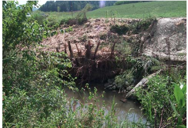
After stream bank repairs to the left bank above cross-section 3, LUS, September 2005.
