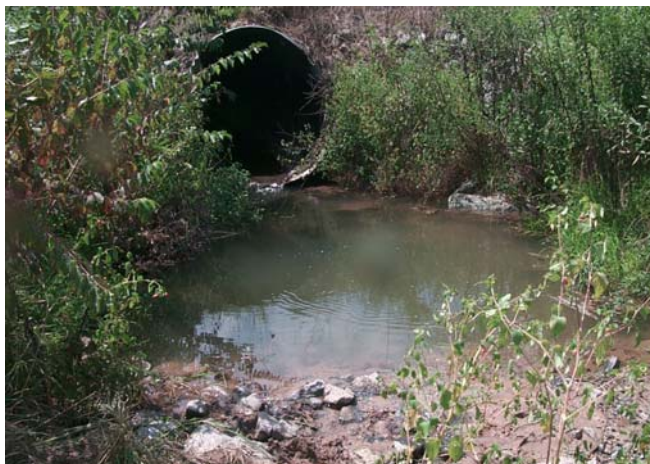
Repositioned boulders and added geotextile fabric to the rock sill in front of the culvert, September 2005.
