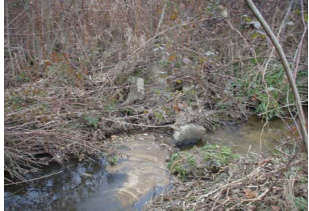
Area in the vicinity of cross-section 2. Water is piping through the boulders November 2008.
