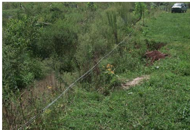
Before stream bank repairs to the left bank around cross-section 3, September 2005.
