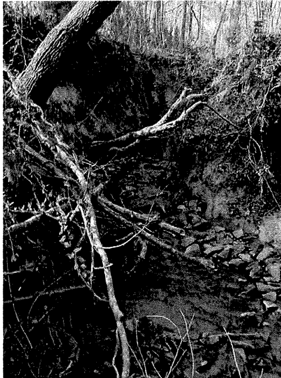
Picture 23. Highly incised and eroded stream banks. Note undercutting and stone that has washed into this area.
