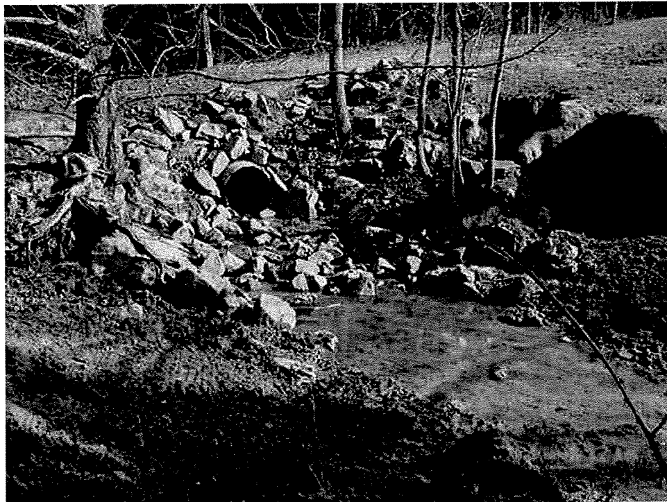
Picture 2. Culvert under farm road at north end of project reach, looking upstream from west bank.
