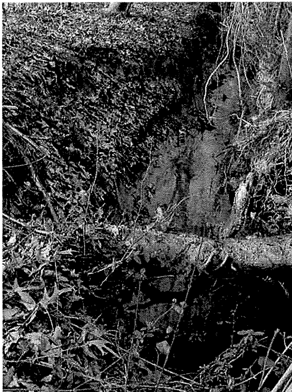
Picture 18. Highly incised banks downstream from fence line shown in Picture 17.
