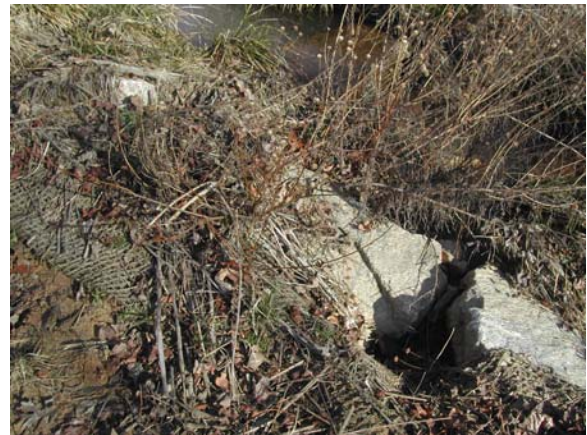
Photo 4: Representative problem rock step structure (Station 15+90 along plan view).
