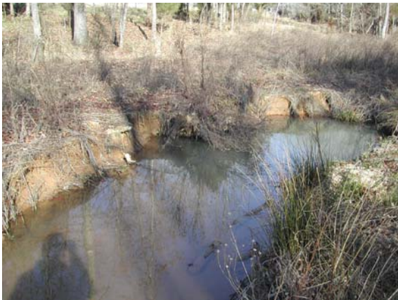
Photo 3: Representative bank erosion problem area (Station 18+82 along plan view).
