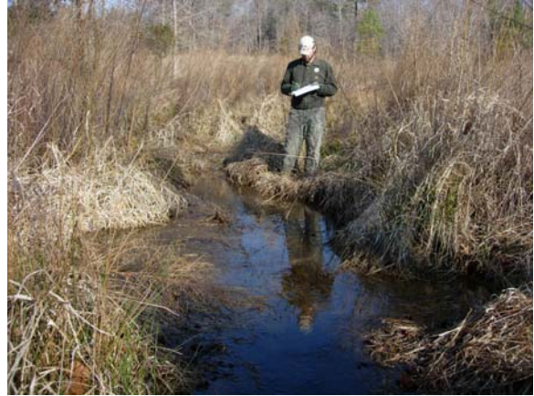
Photo 2: Representative crossvane problem area (Station No. 14+53; view upstream; crossvane is covered in photo; 2-27-2008).
