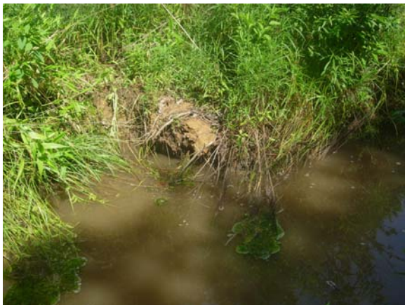
Photo 3: Representative bank erosion problem area (Station No. 18+72; view of right bank; 6-30-2008).
