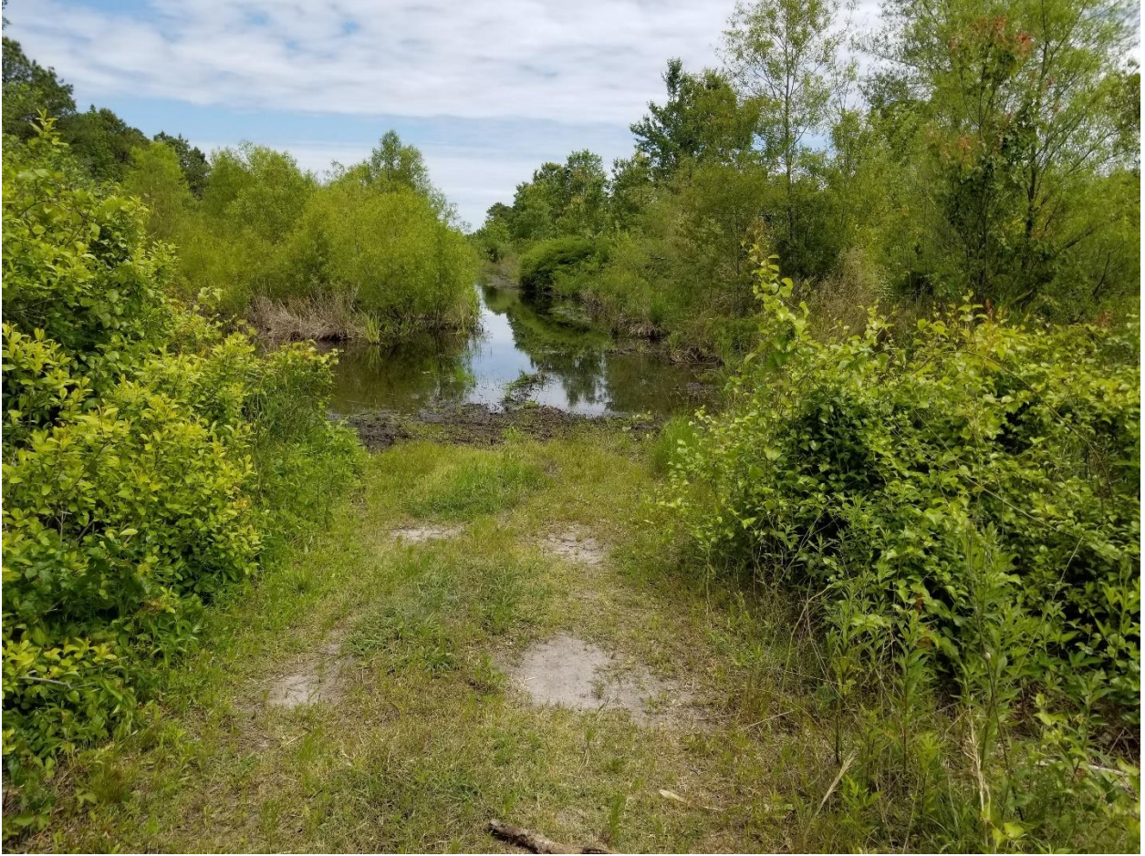
Standing water held by clogged culvert on road in August.
