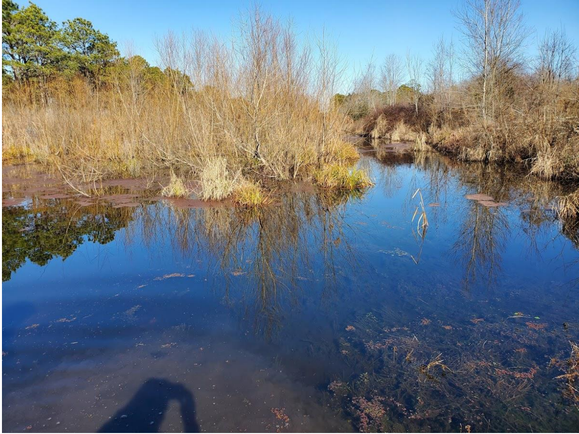
Standing water held by clogged culver on entrance road in January, depth 12".
