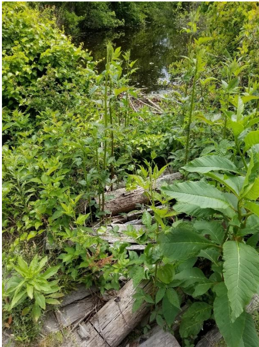
Excessively clogged culvert along entrance road
