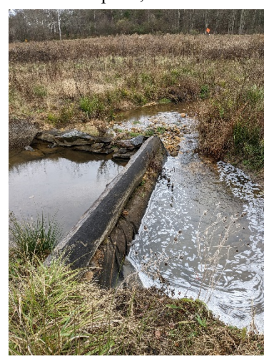
SPA1 (MY1) Before Repair. Photo Taken November 11, 2022 (MY2)
