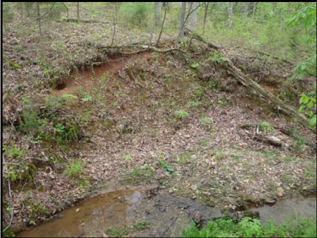
Degrading valley side slope along top of channel bank
