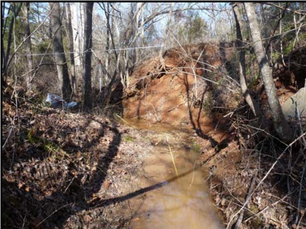
Incised channel with degrading banks
