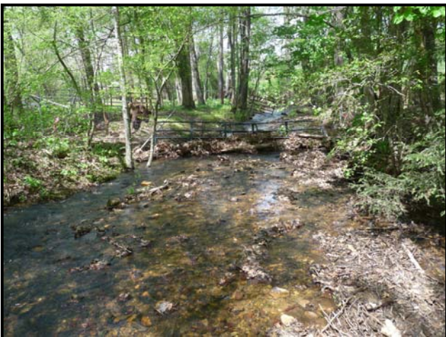
Aggradation and channel widening at fence blockage
