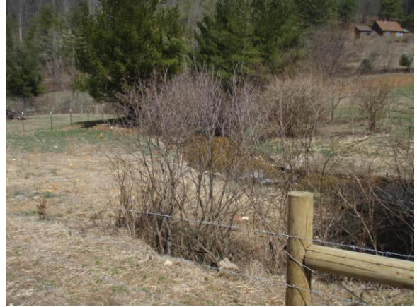
PS-5, bearing 45°: Post-construction view of station 7+25 to station 8+50; 26 Mar 08. Note: stream channel moved to the right.
