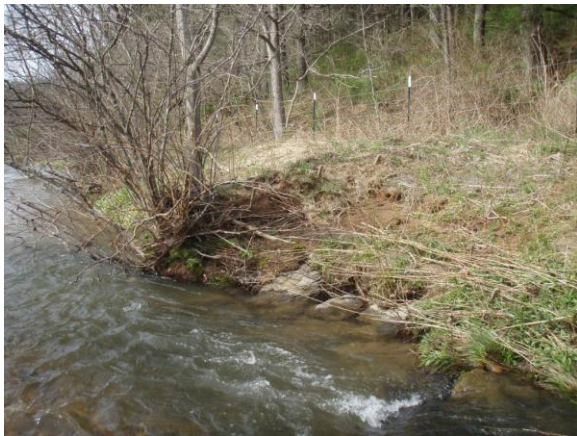
SPA MY4-6, eroding right bank, 19 Apr 11.
