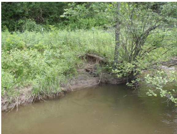
SPA MY5-5, eroding right bank from beaver activity, 21 May 12.
