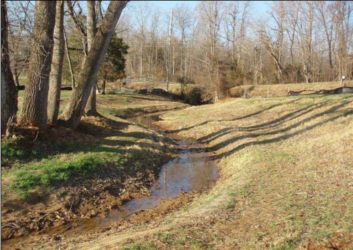
Photo Point 1a: View looking upstream towards the beginning of the project. 12/19/07 – As-Built
