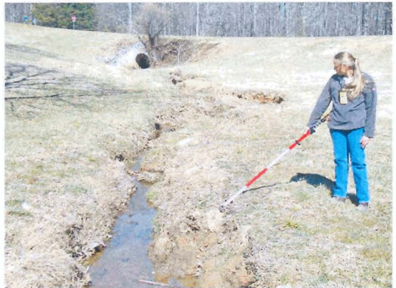
Bank Erosion - Downstream
