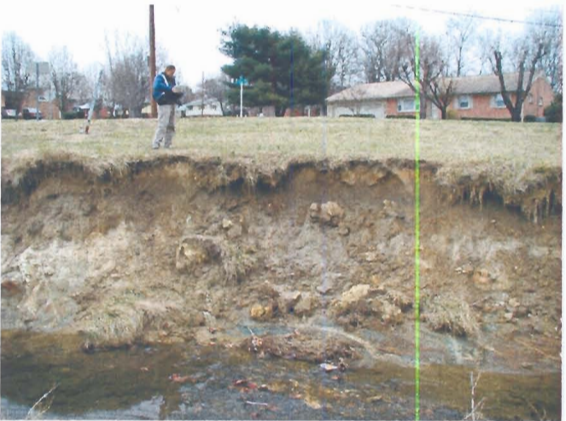
Bank Erosion Downstream
