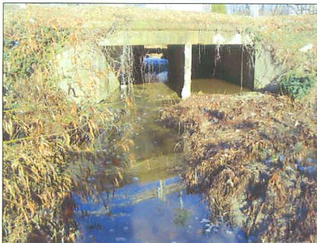
PP#18A R2 upstream view of stabilized culvert from invert of Double Drop Cross Vane #1
