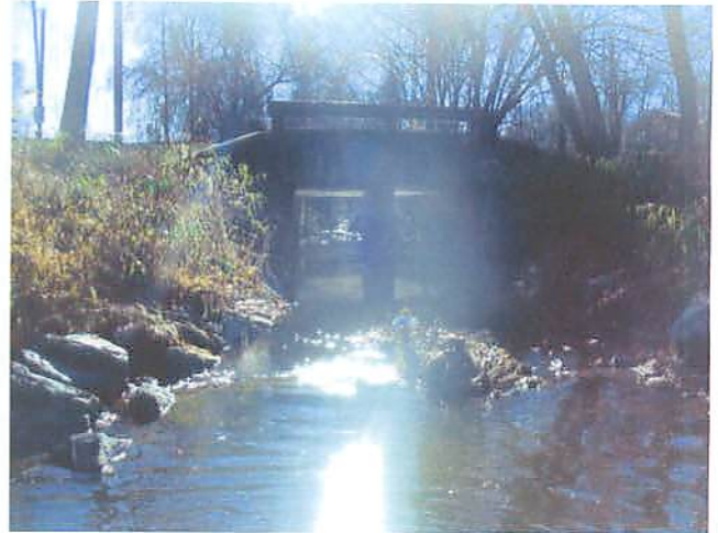
PP#43 R2 Toe protection and rock weir into culvert at end of R2
