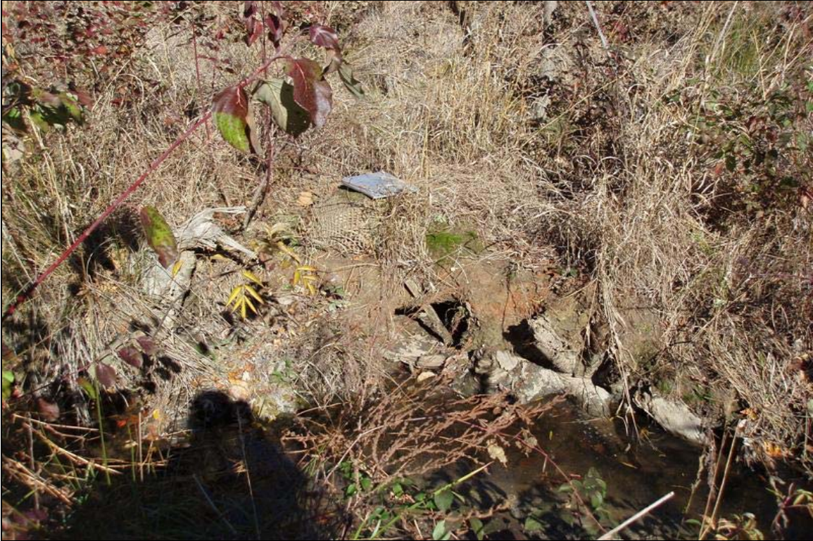
SP1 – Scour behind rootwads under the streambank. Photo taken near Station 18+00. 11/19/07 - MY 03
