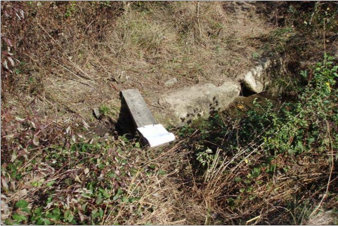
VP3 – The riparian buffer has been cut to create a path. Photo taken near Station 14+20. 10/29/08 - MY 04
