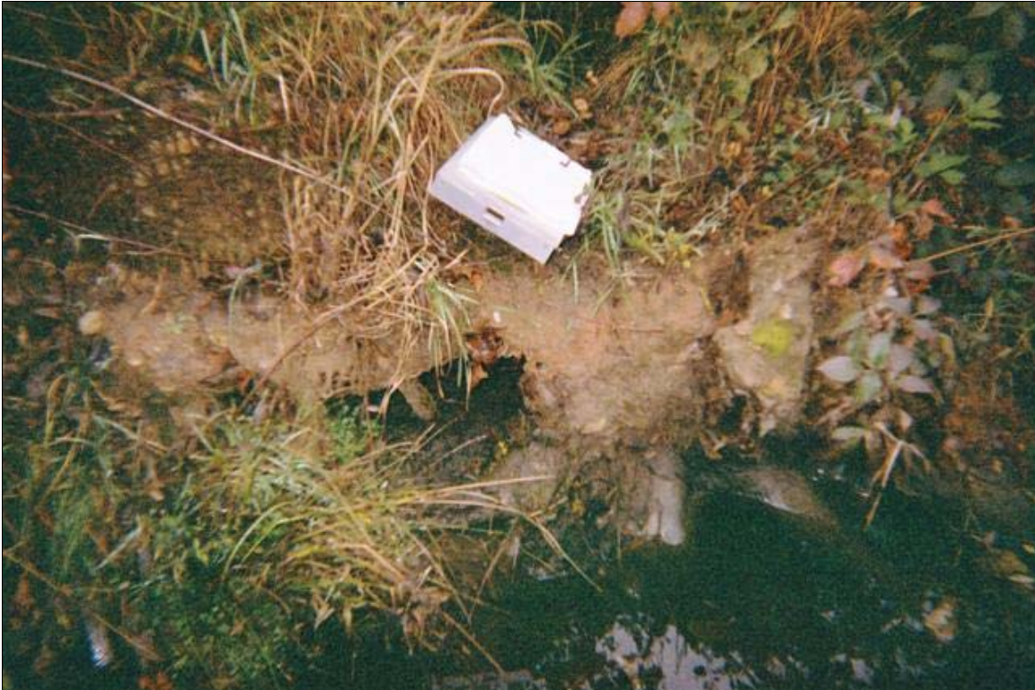
SP1 – Scour behind rootwads under the streambank. Photo taken near Station 18+00. 11/5/08 - MY 04
