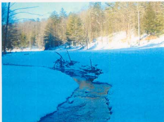
Photograph NM-17. Looking downstream at rock vane, rootwads, and log toe protection from as-built Station ~39+75.
