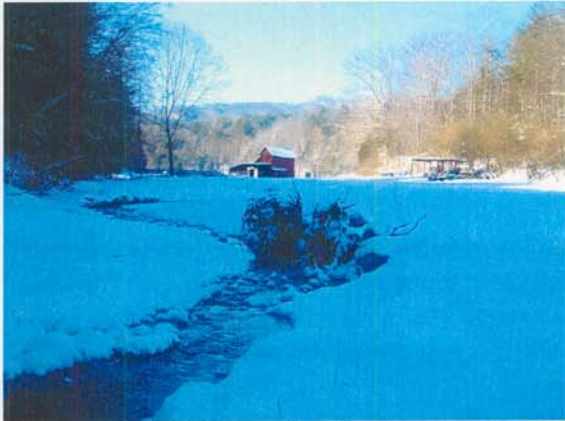
Photograph NM-37. Looking downstream at log toe protection and log vane from Station ~19+70.
