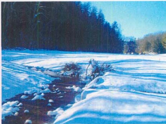
Photograph NM-9. Looking downstream at rootwads and rock toe protection from as-built Station ~43+80.
