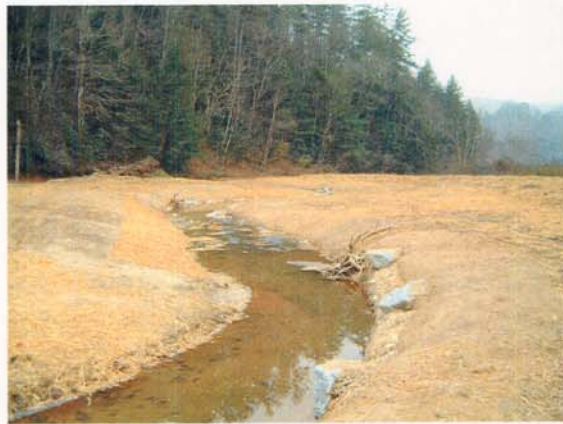
Photograph NM-64. Looking downstream at log toe protection and rootwad from as-built Station ~5+25.
