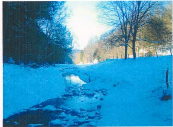
Photograph NM-22. Looking downstream at log vane and log toe protection from as-built Station ~34+00.
