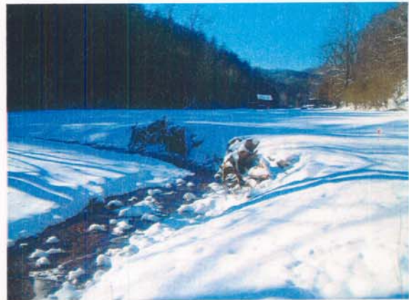
Photograph NM-34. Looking downstream at rootwad and rootwad/log "J" vane from as-built Station ~22+50.
