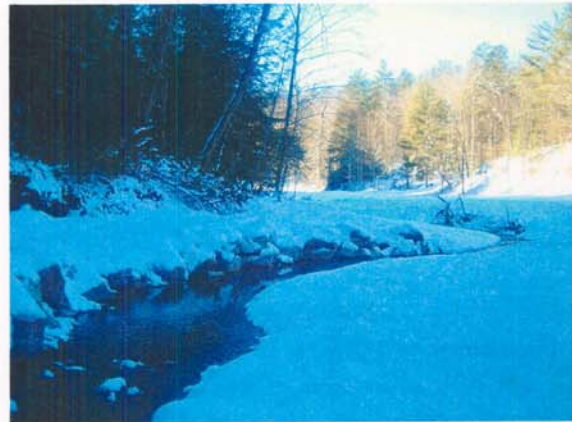
Photograph NM-16. Looking downstream at rock toe protection along opposite bank, view from as-built Station ~41+00.
