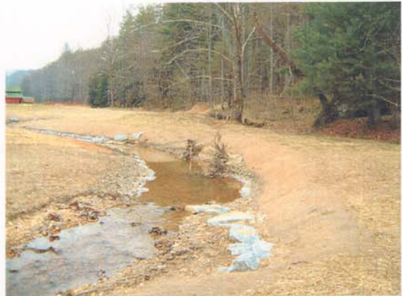
Photograph NM-50. Looking downstream at rock vane and rootwads from as-built Station ~9+50.
