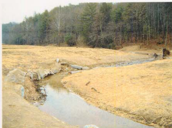
Photograph NM-65. Looking upstream at log toe protection, rootwad, and rock vane from as-built Station ~4+50.
