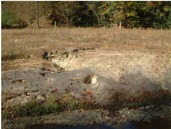
Gully erosion on right bank at as-built Station ~21+75.
