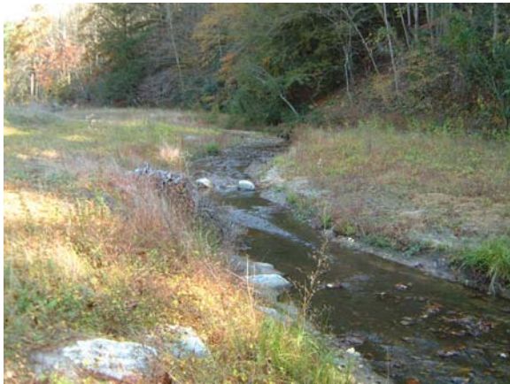
Photograph NM-75. Looking upstream at rock vane and rootwad from as-built Station ~0+65.
