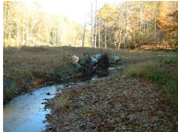
Looking upstream at lateral channel movement and erosion at as-built Station ~19+00.
