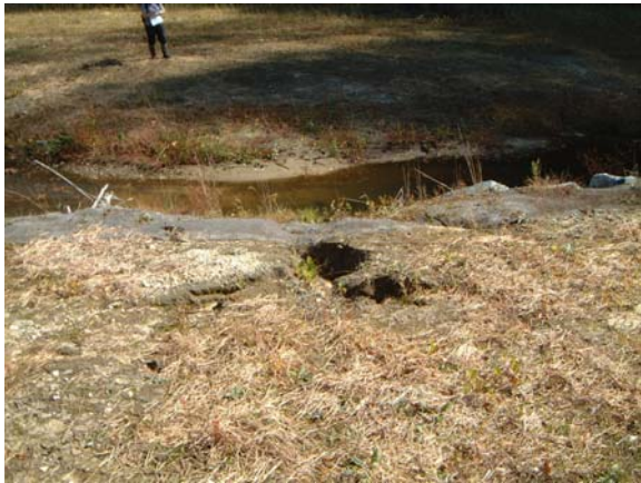
Looking downstream at gully erosion at as-built Station ~3+00.
