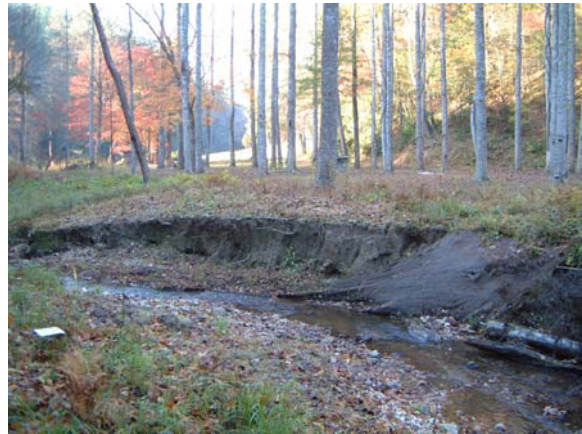
Looking downstream at bank erosion from as-built Station ~47+00.
