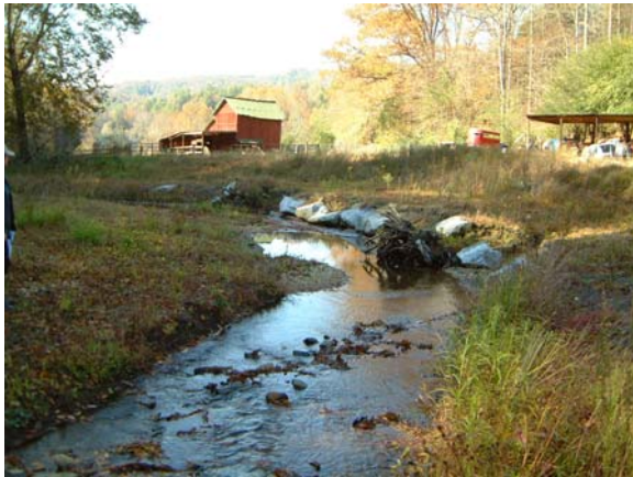
Photograph NM-39. Looking downstream at log vane and rootwad from as-built Station ~17+75.
