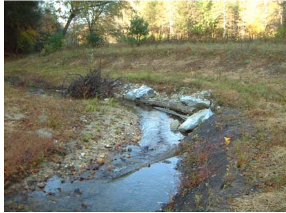
Photograph NM-20. Looking downstream at log vane, rootwad, and log toe protection from as-built Station ~36+25.
