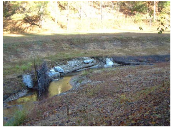
Looking upstream at bank erosion at as-built Station ~36+00.
