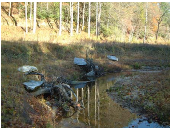
Looking upstream at erosion behind rootwads at as-built Station ~24+00.
