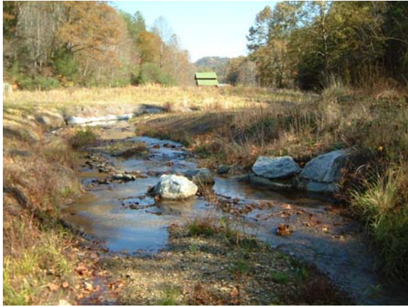
Looking upstream at channel widening and rock "J" vane from as-built Station ~10+25.
