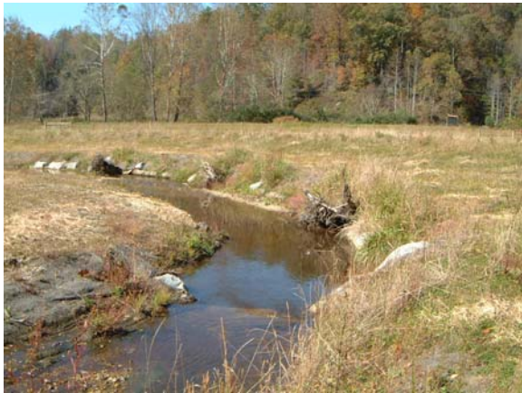
Photograph NM-51. Looking downstream at cross vane and rootwads from as-built Station ~9+00.
