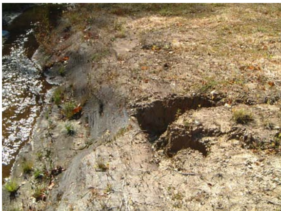
Looking downstream at gully erosion at as-built Station ~7+25.
