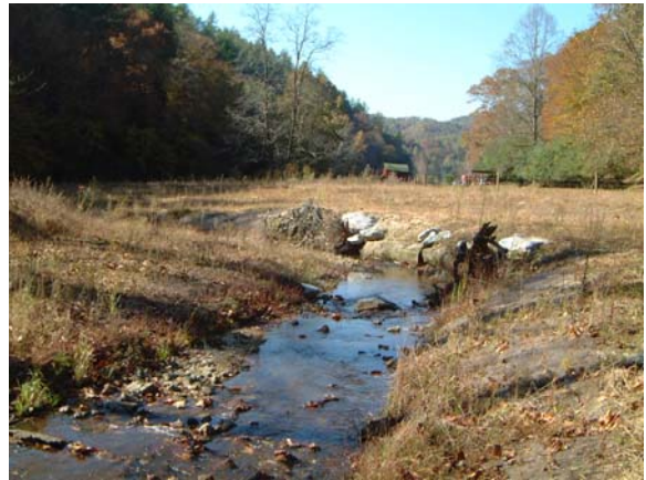
Photograph NM-34. Looking downstream at rootwad and rootwad/log "J" vane from as-built Station ~22+50.
