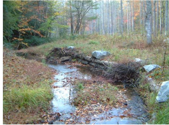
Photograph NM-2. Looking downstream at rootwads and log toe protection from as-built Station ~51+00.
