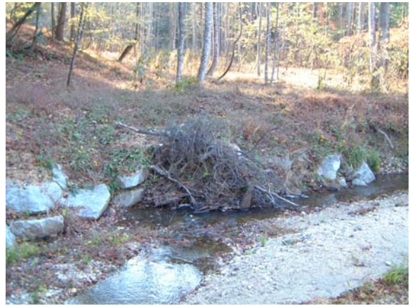
Photograph NM-8. Looking downstream at rootwad and rock toe protection from pedestrian bridge at as-built Station ~44+60.
