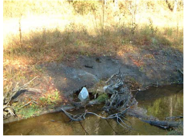
Looking upstream at erosion behind rootwads from as-built Station ~29+90.
