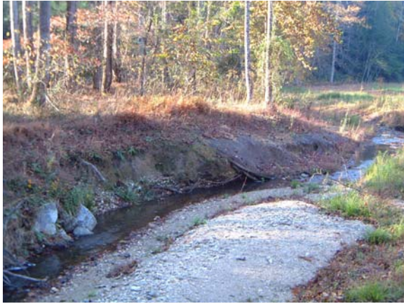
Looking downstream at erosion from as-built Station ~44+00.
