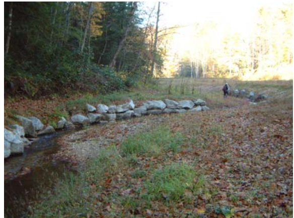
Photograph NM-16. Looking downstream at channel plug protection along opposite bank, view from as-built Station ~41+00.
