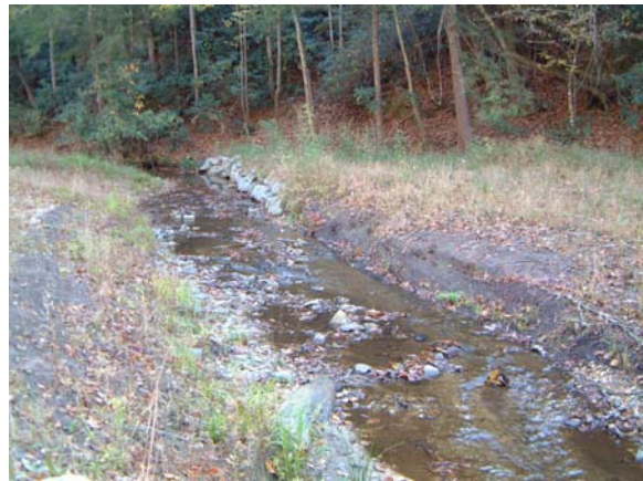
Photograph NM-30. Looking upstream at log vane and rock toe protection from as-built Station ~24+60.
