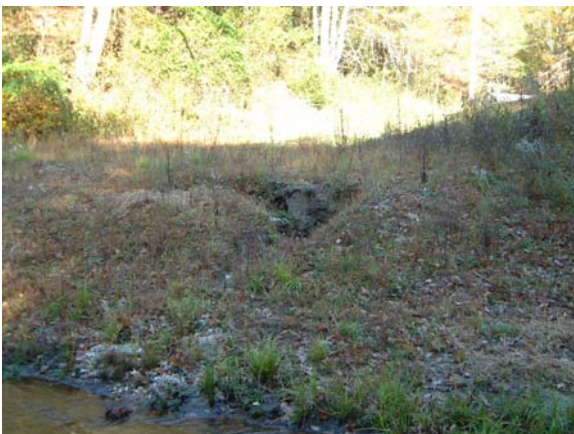
Looking downstream at gully erosion at as-built Station ~31+10.
