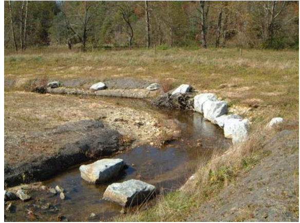
Photograph NM-62. Looking downstream at rock "J" vane, rock toe protection, and rootwad from as-built Station ~5+50.
