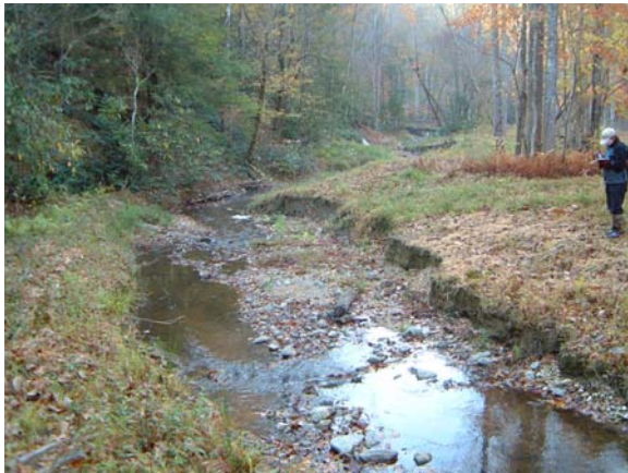
Looking downstream at bank erosion from as-built Station ~49+25.
