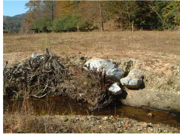
Looking downstream at erosion behind rootwads at as-built Station ~22+00.
