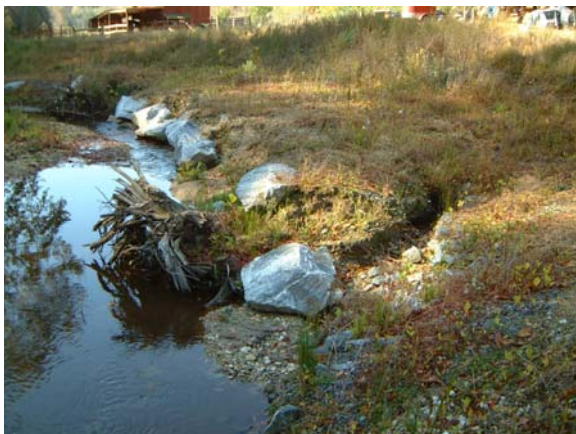
Looking downstream gully erosion at as-built Station ~17+25.
