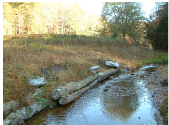
Looking upstream at slumping log wall at as-built Station ~30+50.
