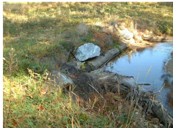
Looking upstream at erosion behind rootwad at as-built Station ~14+00.
