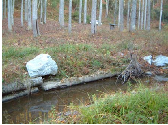
Looking upstream at log wall damage from as-built Station ~49+00.
