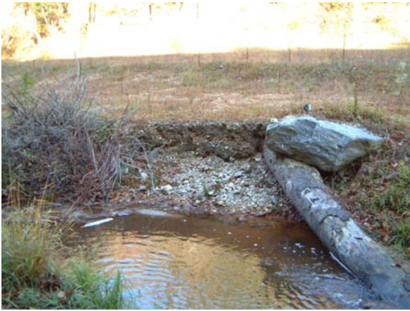
Looking downstream at erosion between rootwad and log vane at as-built Station ~36+00.
