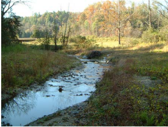
Photograph NM-73. Looking downstream at rock “J” vane and rootwad from as-built Station ~1+00.
