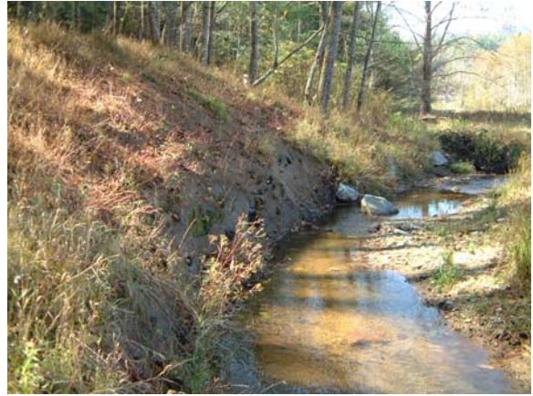
Looking downstream at erosion on left bank from as-built Station ~12+50.
