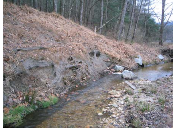
Issue Photo 4 Bank Erosion at STA: 38+50
