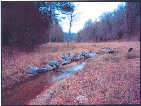
STA 18+50 Looking Downstream @Failing Boulder Bar
