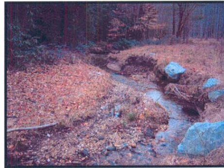
STA 0+30 Bank Erosion Right Bank Looking Downstream
