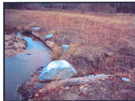
STA 46+20 Looking Downstream @Failing Root Wad
