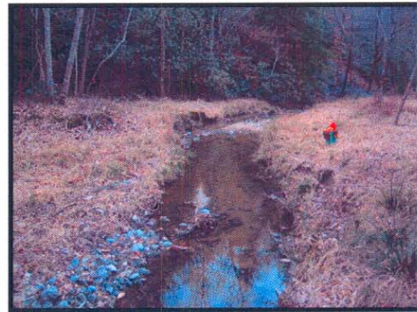
STA 2+00 Bank Erosion Looking Downstream
