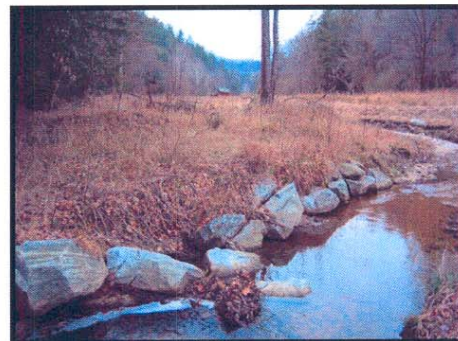
STA 25+90 Looking Downstream @Failing Boulder Wall
