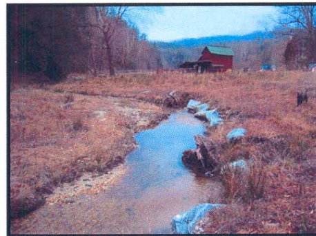
STA 33+25 Looking Downstream @Bank Erosion
