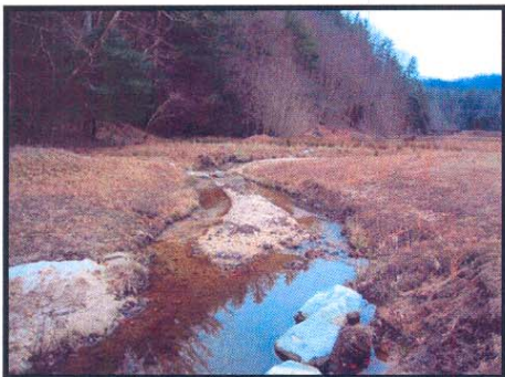
STA 39+90 Downstream @ Mid-Channel and Bank Erosion
