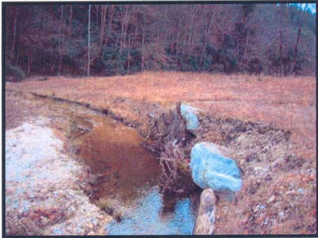
STA 28+50 Looking Downstream @ Bank Erosion Tight Radius of Curvature
