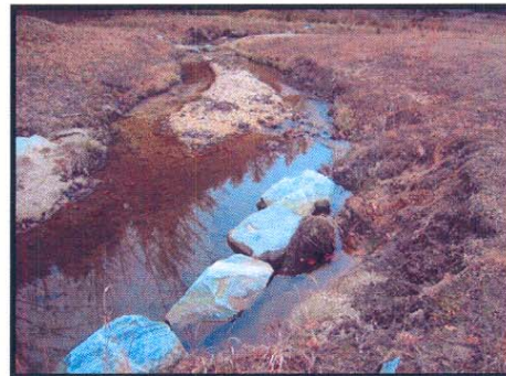
STA 39+90 Downstream Erosion
