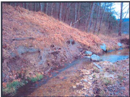
STA 38+50 Looking Downstream @ Valley Bank Erosion
