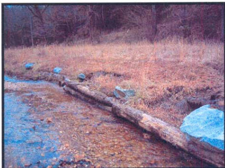
STA 20+70 Looking Downstream @Exposed Toe Log
