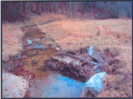
STA 36+90 Downstream @ Bank Erosion
