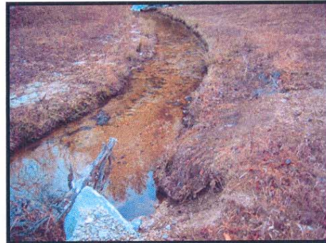
STA 29+00 Looking Downstream @Bank Erosion
