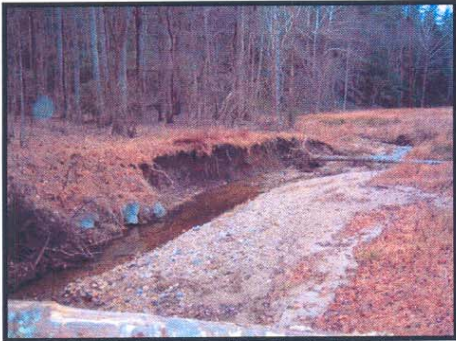
STA 6+75 Bank Erosion Left Bank Looking Downstream
