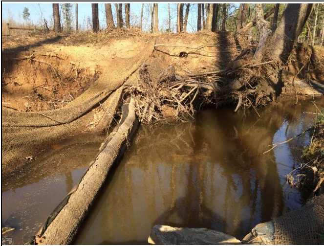
1) Reach UT4-R3 – Log vane failure and bank erosion at Station 29+00
