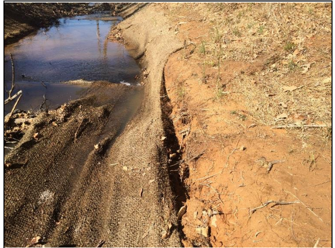
2) Reach UT4-R2 – Bank erosion at Station 37+40
