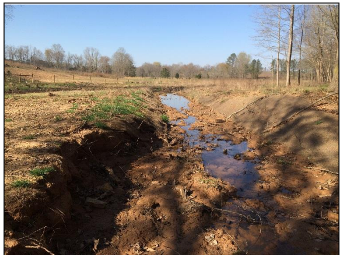
6) Reach UT4-R2 – Riffle scour at Station 24+00, and bank scour/mass wasting at Station 23+10
