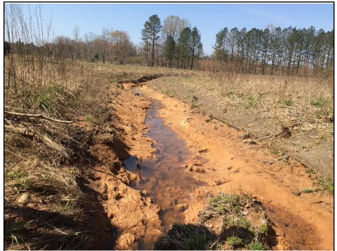
4) Reach UT4-R2 – Riffle scour at Station 31+00
