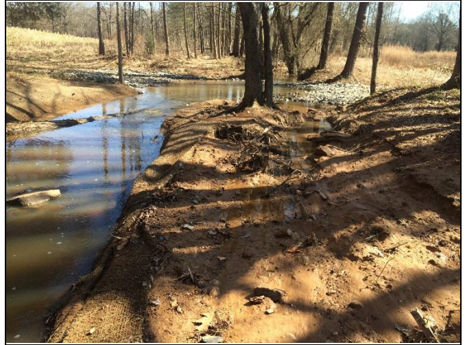
8) Reach UT4-R2 – Scour in floodplain, view upstream, Station 22+00
