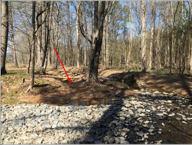
7) Reach UT4-R2 – Scour in floodplain, view downstream, Station 21+25
