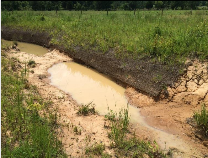
1) Reach UT4-R2: Bank erosion at Station 31+75
