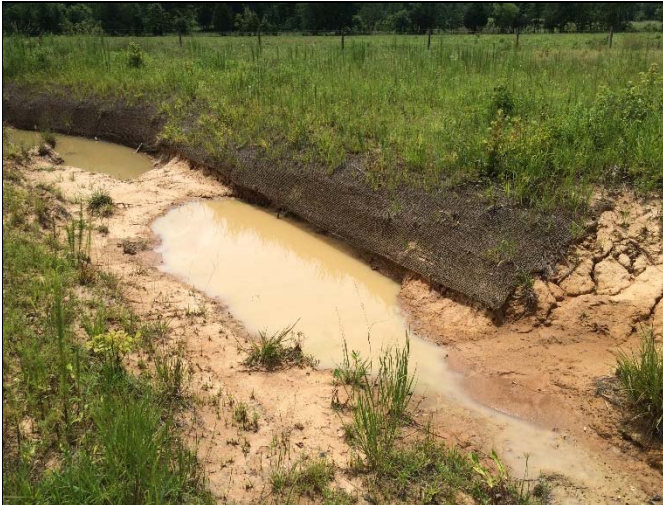
1) Reach UT4-R2: Bank Erosion, Station 31+75 (BEFORE)
