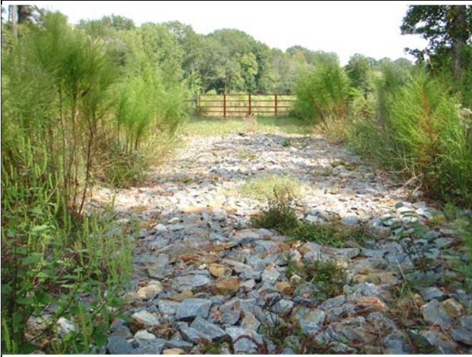
1) Reach UT4-R4b: Rock crossing, Station 25+30
