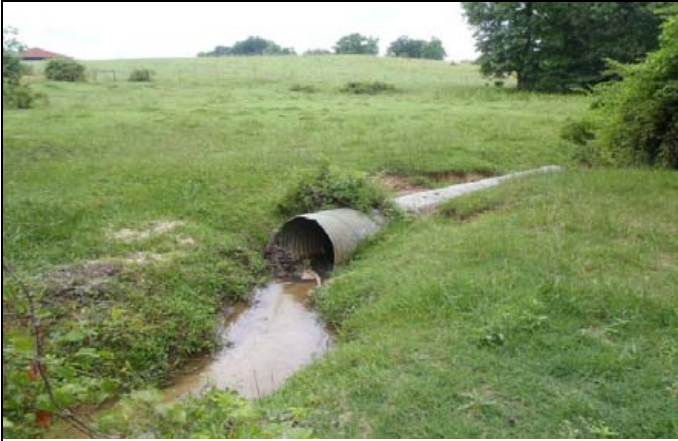
Culvert acting as cattle crossing at upper end of Reach R1. This culvert will be removed. (6/4/13)
