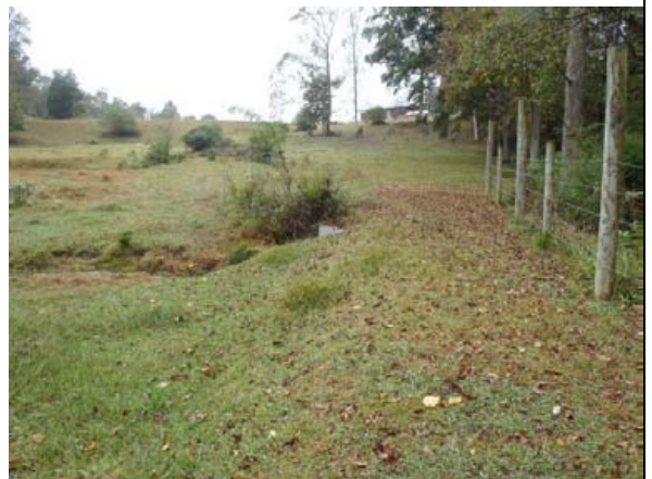
Culvert at downstream end of project will be replaced and the dam will be enhanced to prevent piping. (10/10/13)
