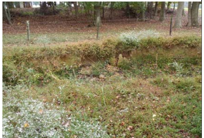
Unstable section of Reach R3 showing vertical banks and lack of floodplain access, mass wasting/failing streambank, and lack of riparian buffer. (10/17/13)
