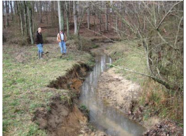
View looking upstream along Reach R2 at bank erosion on right bank and lack of riparian buffer. (2/27/12)
