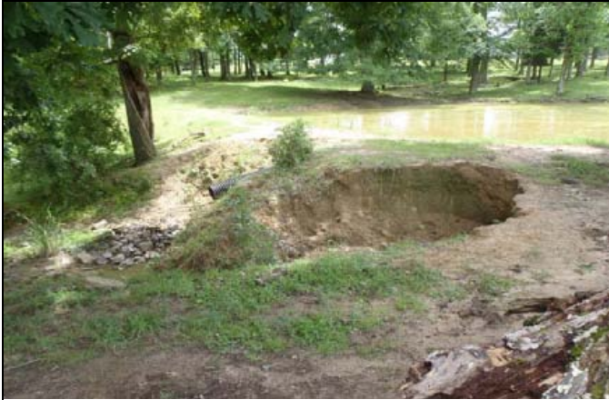
Lower end of pond on Reach R4. Headcut threatens pond dam. Pond will be removed as part of restoration. (9/10/13)
