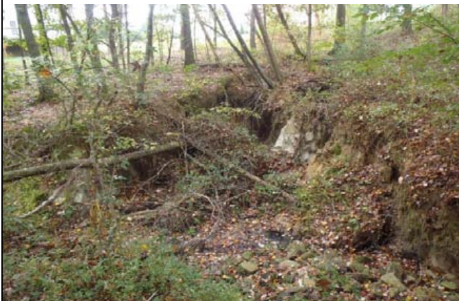
Right bank along Reach R4 where stormwater inputs from Broad Ridge Ct. have initiated a headcut. (10/17/13)
