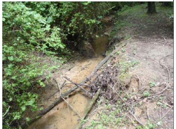
View looking downstream along Reach R2 shows active erosion and deficient riparian buffer. (6/4/13)
