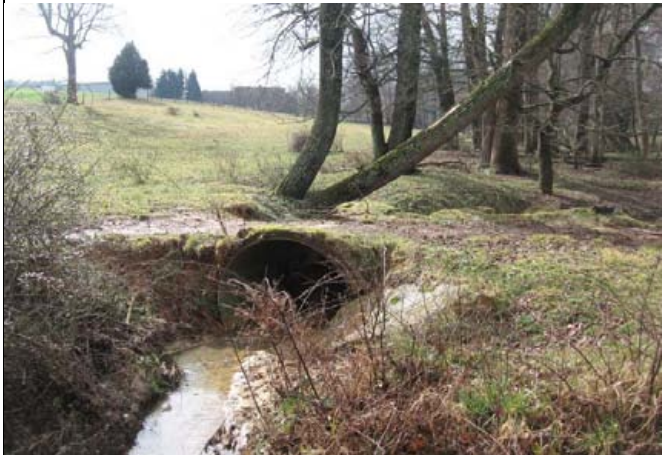
Existing stream crossing on Reach R3. This culvert will be replaced and the crossing will be widened. (2/27/12)
