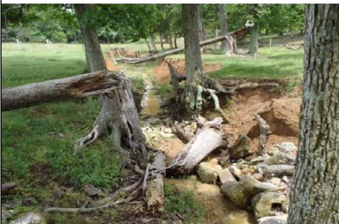
View looking downstream down Reach R6. Concrete and other debris have been placed to stop headcut migration. (6/4/13)
