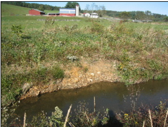
Issue Photo 3. Little Pine near station 6+50. Bank Scour on Right Bank
