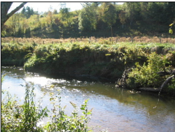
Issue Photo 1. Brush Creek near Station 2+00. Right bank slump and scour.
