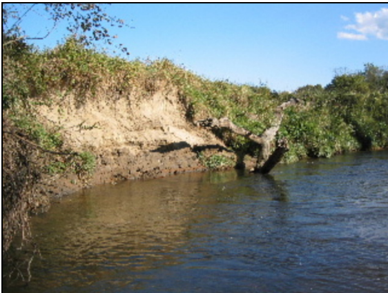
Issue Photo 1. Brush Creek near Station 1+50. Left Bank slump and scour.
