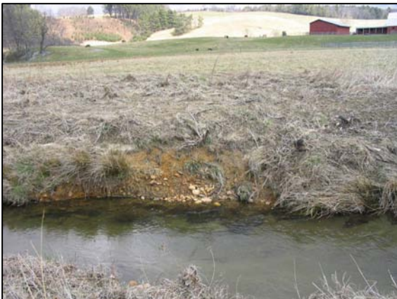
Issue Photo 3. Little Pine near station 7+80. Bank Scour on Right Bank
