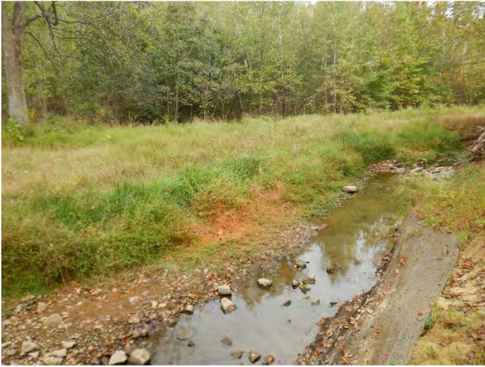
Before - Localized Erosion (10/9/2019)
