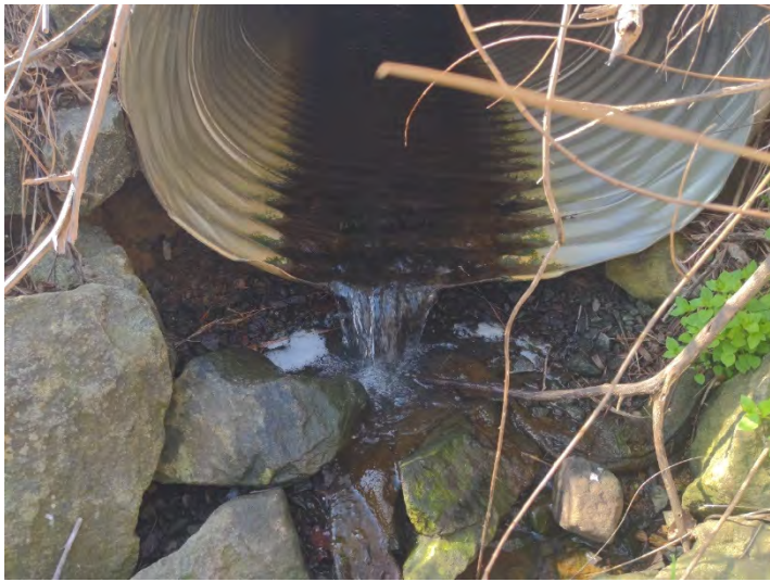
T4 STA 408+42 – Perched Culvert (3/24/2023)
