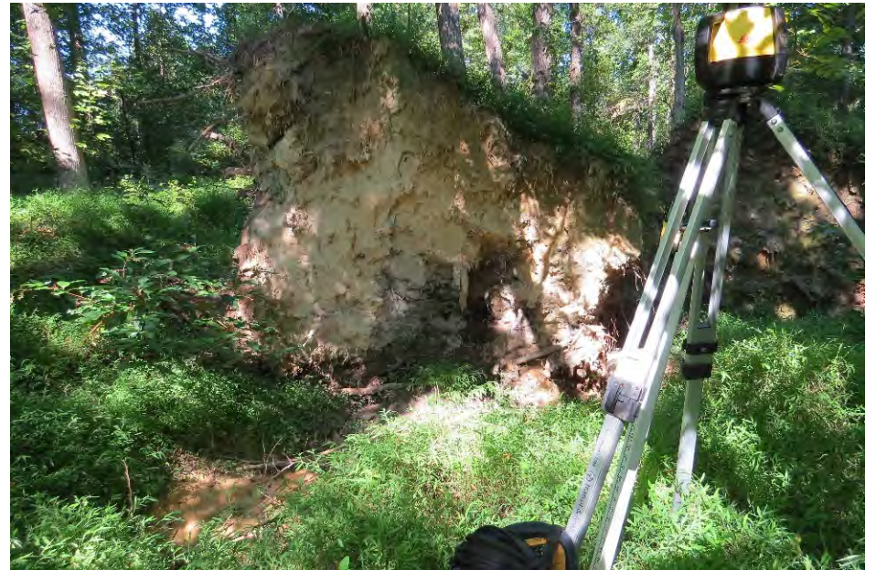
Reach R6 – Erosion of spoil piles along R6
