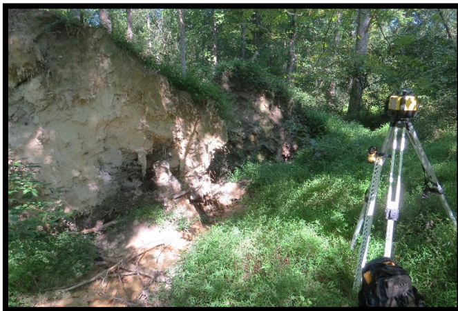
Looking downstream below pond at poor channel definition and stream bank erosion along R6.
