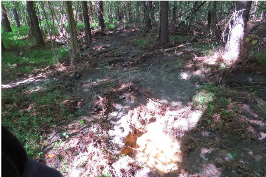
Erosion from stormwater outfall adjacent to Reach R5
