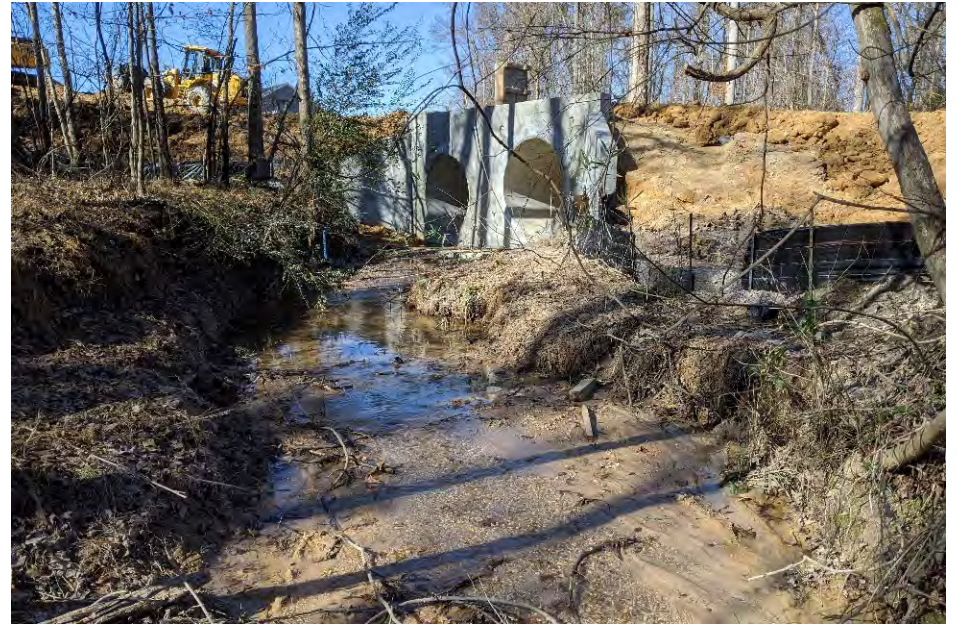
Reach MS-R2 – Sedimentation downstream of new culvert
