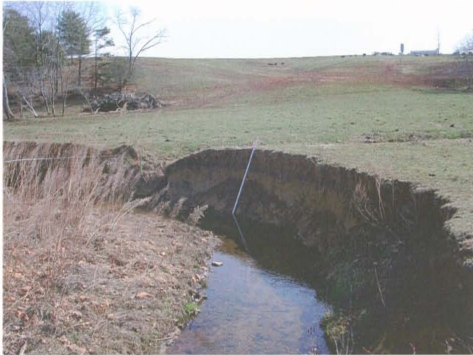
Picture 5. Pool cross-section at severely eroding meander on Little Bugaboo Creek. Looking downstream.
