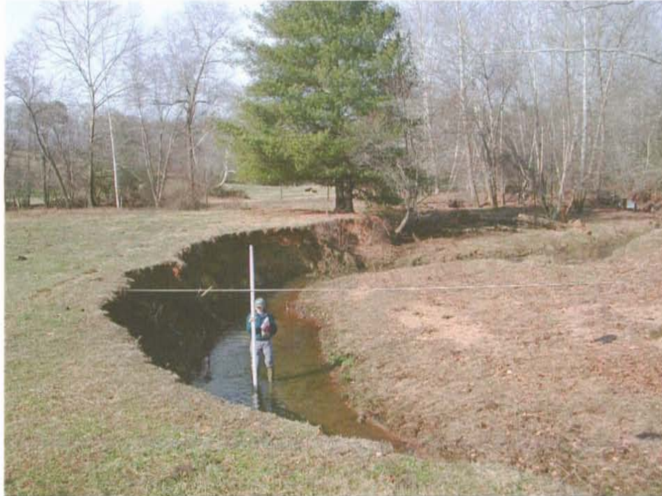
Picture 4. Pool cross-section at severely eroding meander on Little Bugaboo Creek.
