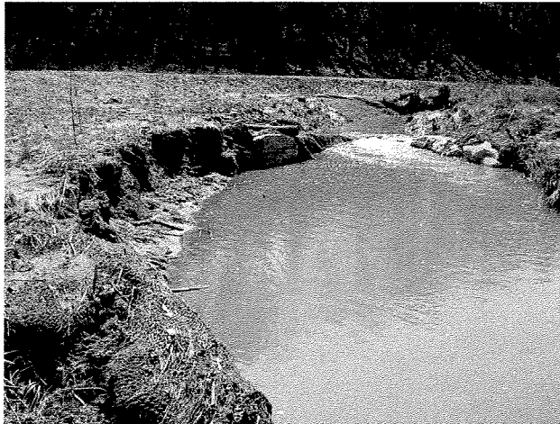
Lack of vegetation, leading to bank erosion also triggered by eddy downstream of structure (bowling effect).
