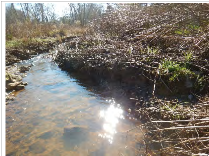
Before – Localized Toe Erosion (11/17/2022)
