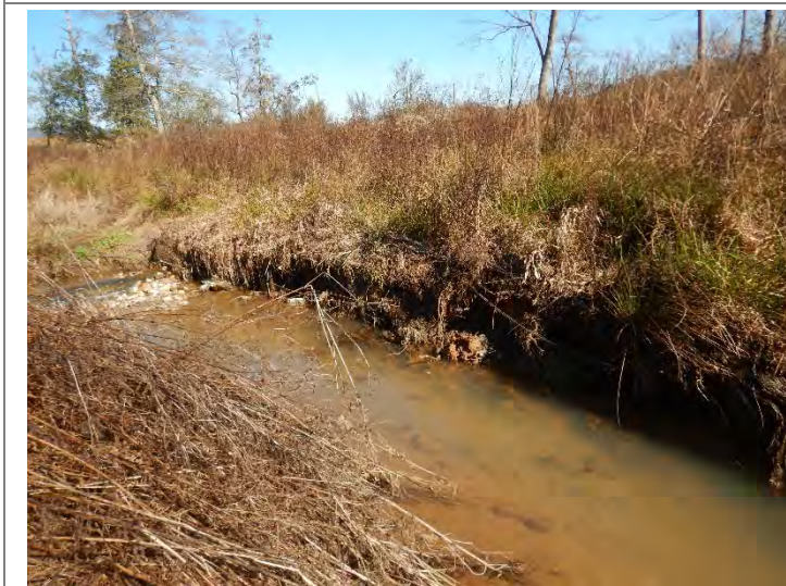
Before – Localized Toe Erosion (11/17/2022)
