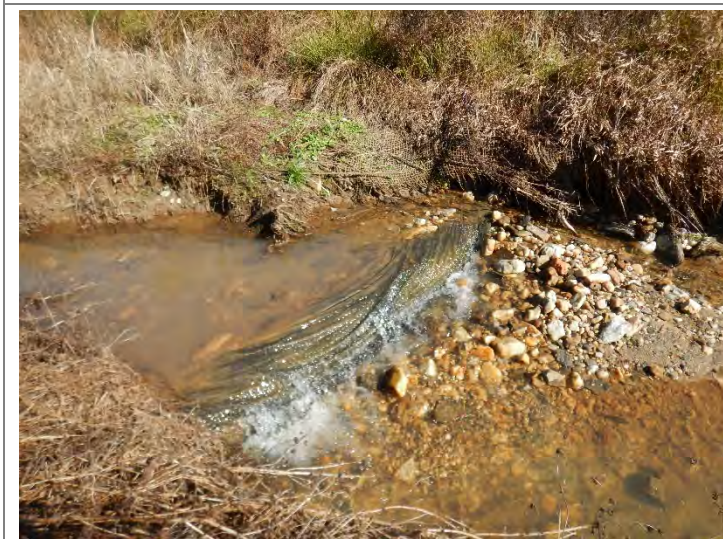
Before – Eroded Log Sill at STA 139+59 (11/17/2022)
