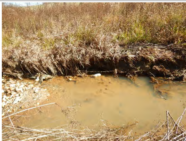
Before – Localized Toe Erosion (11/17/2022)
