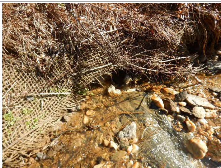
Before – Eroded Log Sill at STA 139+59 (11/17/2022)
