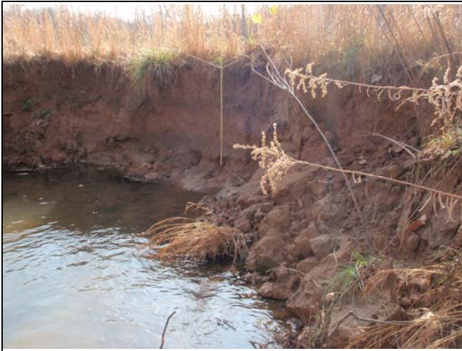
Severe bank failure on mainstem
