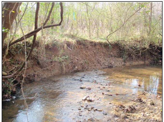
Near vertical banks on mainstem
