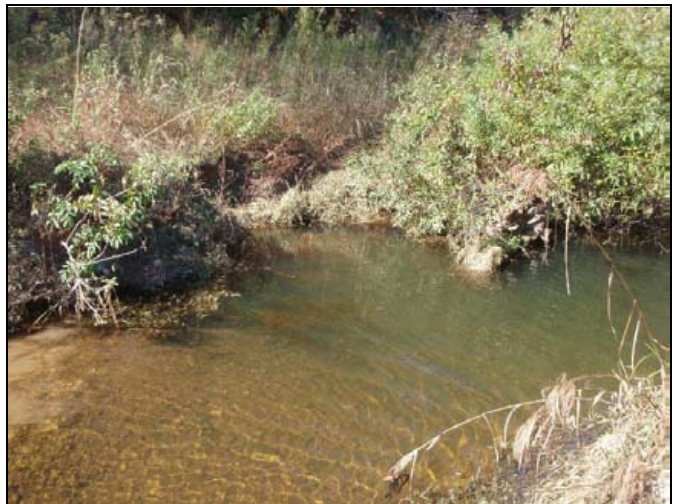
Stream Problem Area 2 - STA 55+50. M3 bank erosion on outer portion of meander bend.
