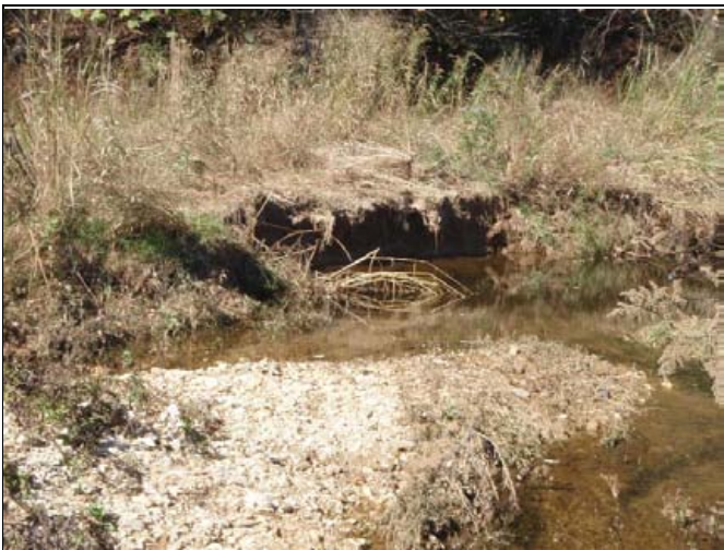
Stream Problem Area 1 - STA 46+50. M3 bank erosion on outer portion of meander bend.
