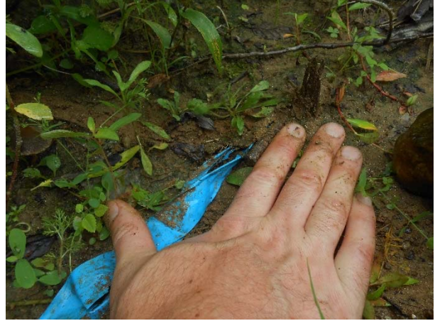
Top Bank Pin – Reach M1, right bank Between Station 11+00 and 12+00 August 14, 2017
